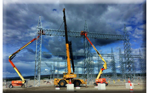
Finalizing installation of steel gantry towers at Bottom Brook site, NL for the Maritime Link Project.
