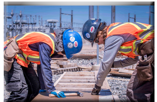
Two apprentice carpenters work at Woodbine site, NS for the Maritime Link Project
