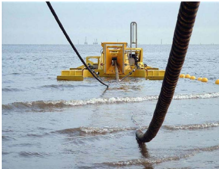
Figure 9.5: Sea Stallion 4 Cable Plow Burying North Hoyle Export Cables up the Beach (Photo courtesy of The Engineering Business Ltd)
