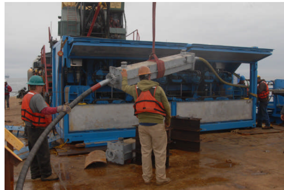
Figure A.8: Splice box rigged and ready
