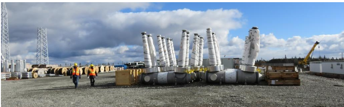
Photo 32 - Woodbine – ABB circuit breakers awaiting installation in switchyard. Spools of cable and other materials located at left side of photo.
