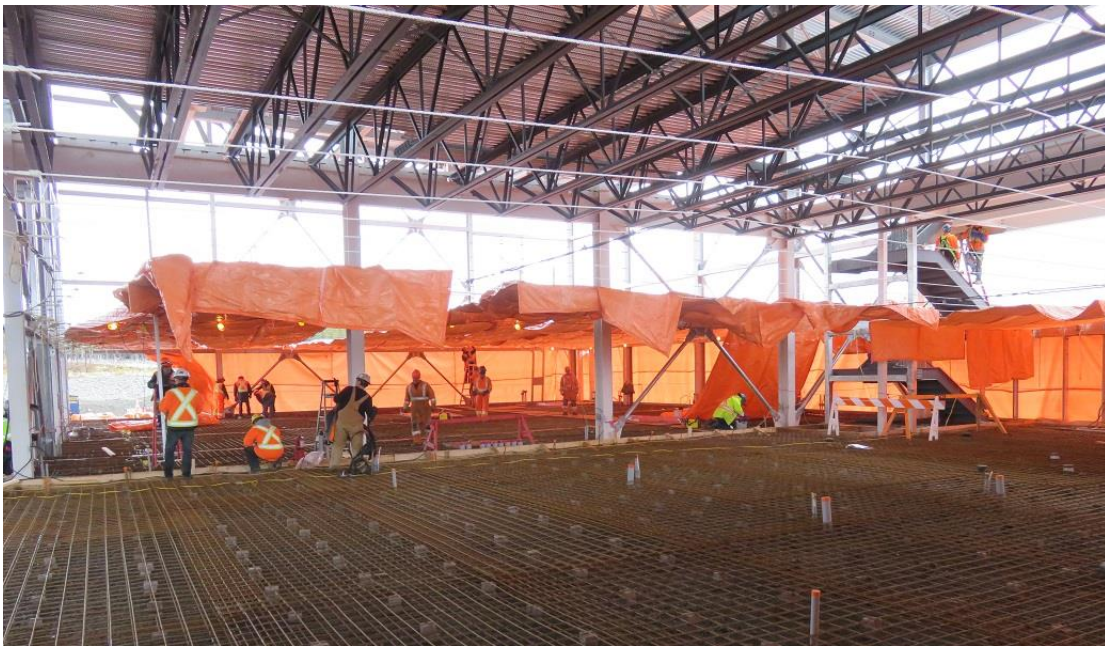
Photo 2 - Bottom Brook – welded wire fabric reinforcement installed in preparation for converter building concrete floor slab placement. Insulated tarps are being installed in background to maintain adequate temperature for concrete curing. Roof trusses and Q deck roof visible at top of photo.
