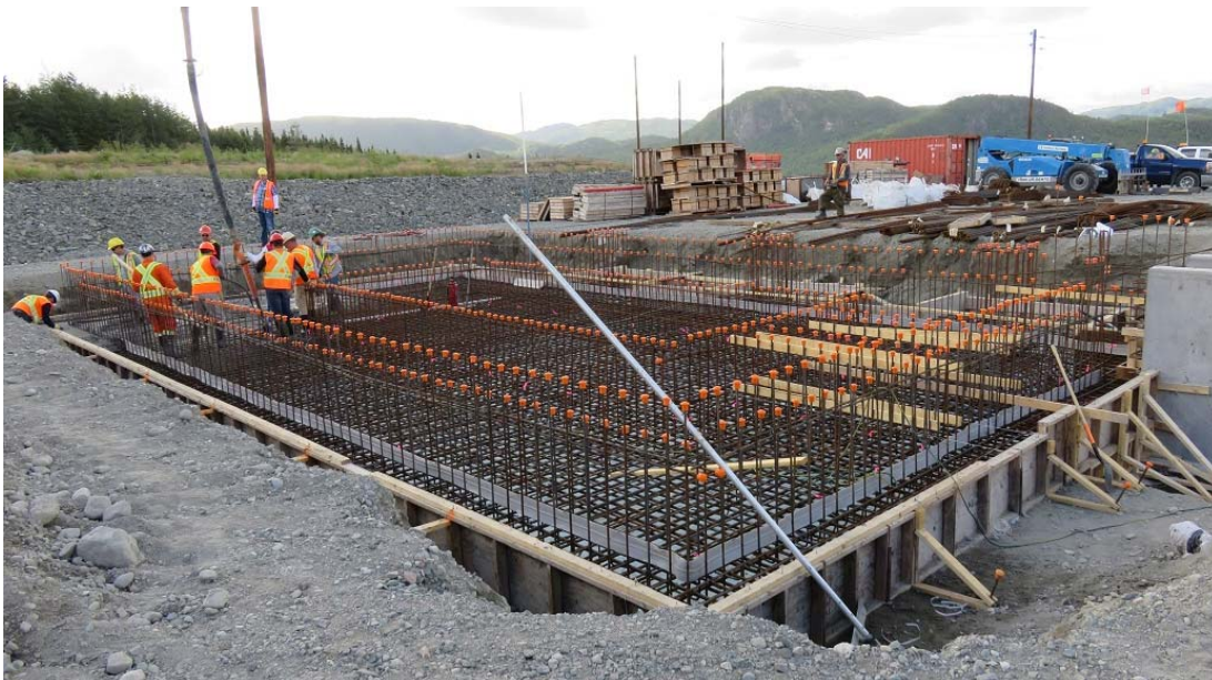
Photo 15 - Bottom Brook – concrete placement in progress for converter transformer foundation. Note safety caps on exposed vertical rebar ends.
