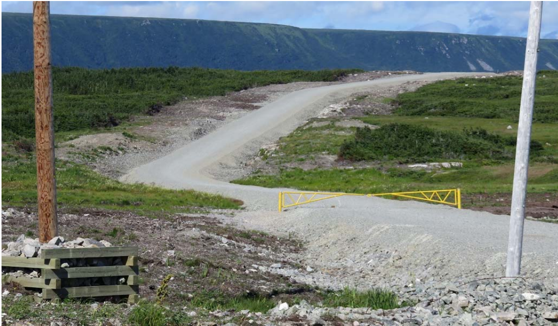
Photo 10 - Cape Ray – view from HDD site looking up completed access road to the transition compound site. The HVDC line between the HDD site and the transition compound will be buried beside the road.
