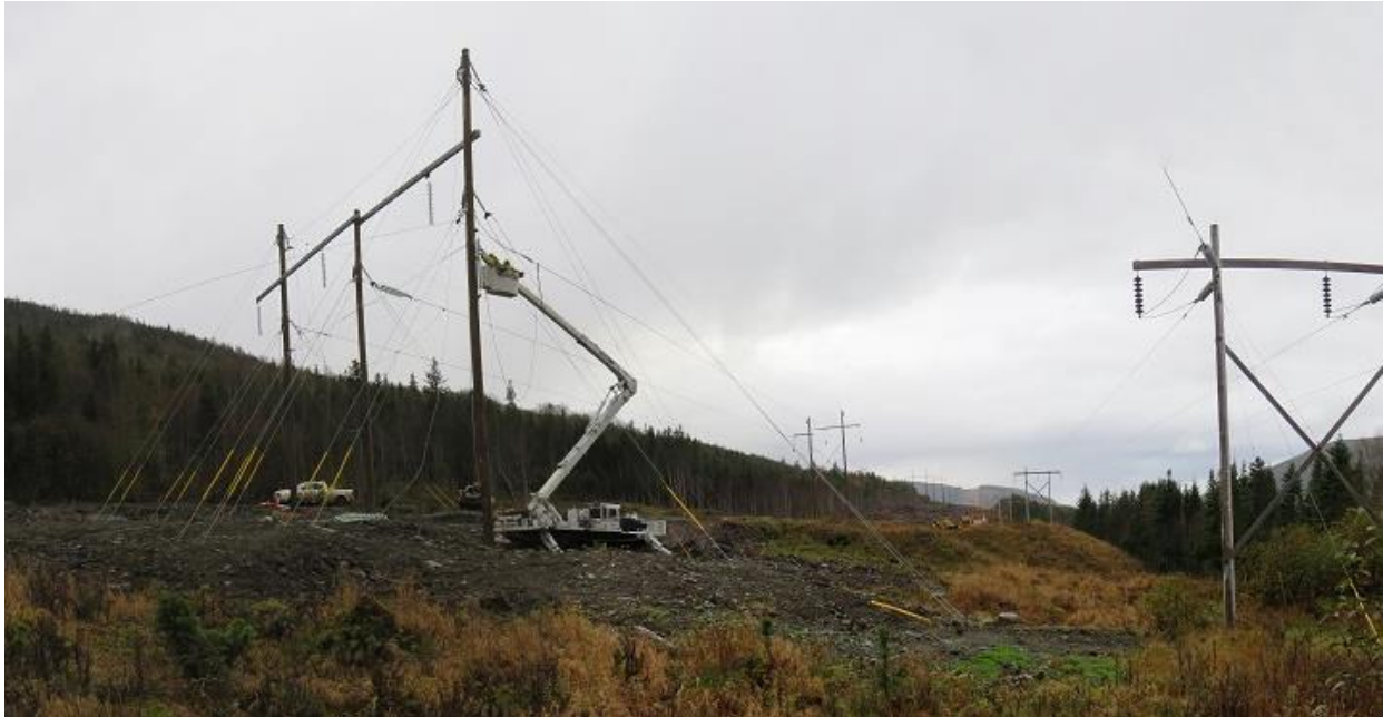
Photo 16 - Westerly view along HVAC line along Burgeo Highway, with Tower 259 at left. Line tensioning of section to Tower 280 is in progress. Existing line at right.
