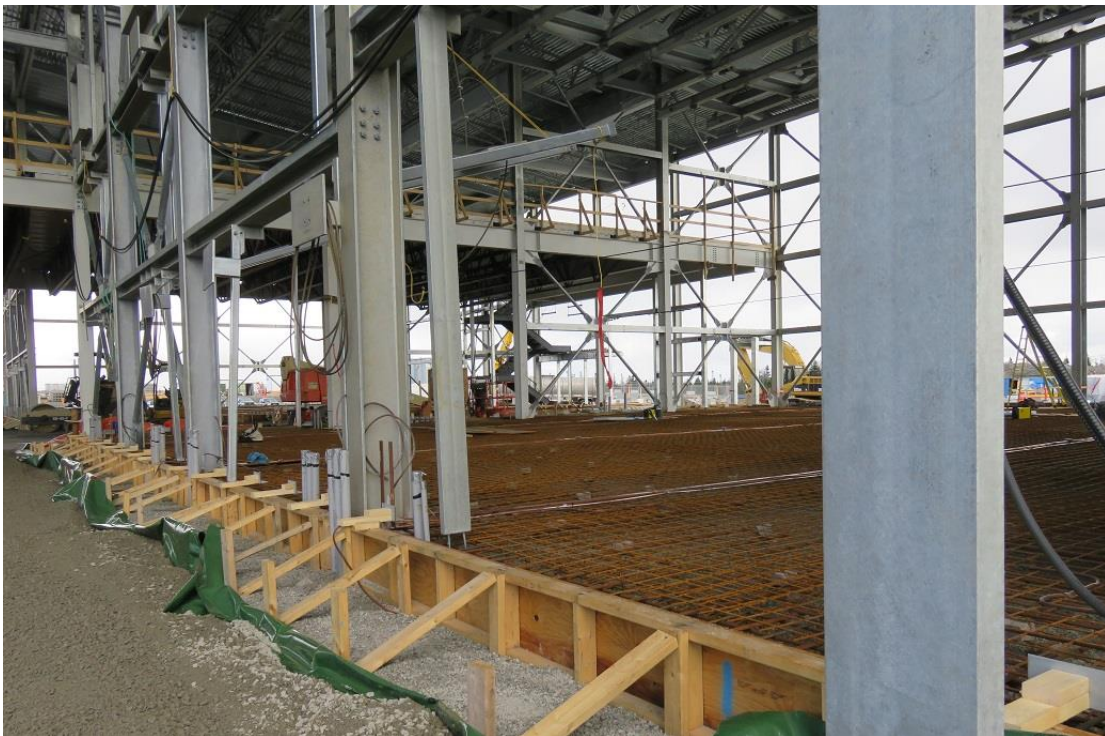
Photo 30 - Woodbine – interior of converter building with concrete floor reinforcement in place in some areas.
