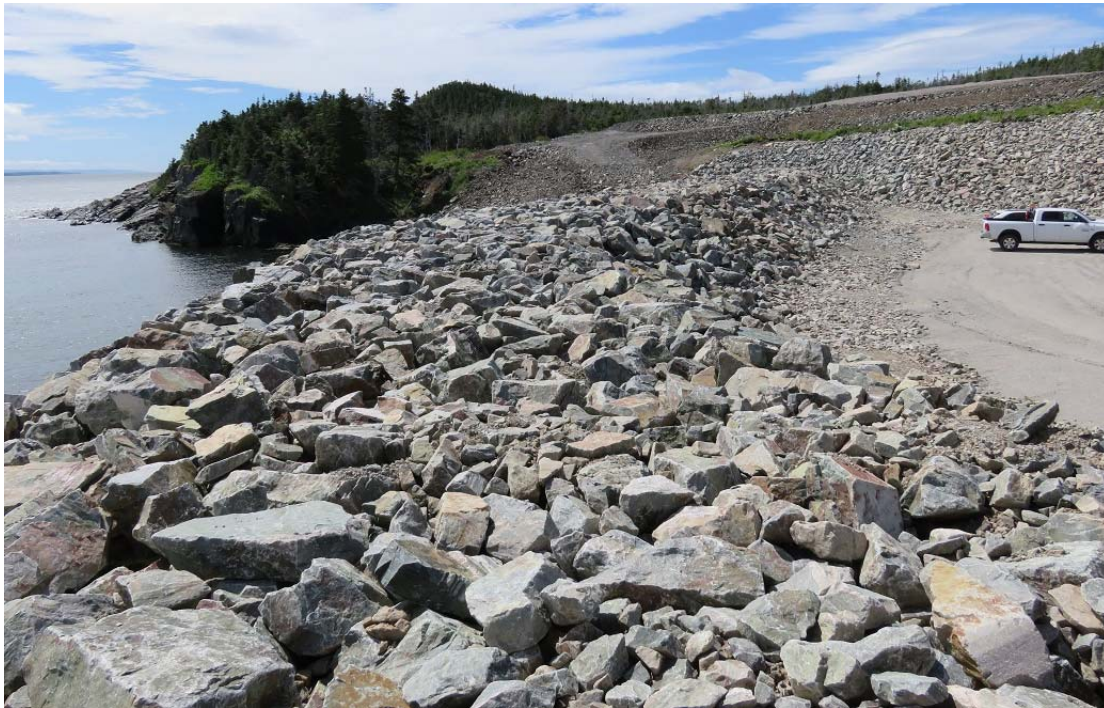
Photo 6 - Indian Head Grounding Site – Protective rock berm constructed in water. Construction access road in background has been decommissioned.
