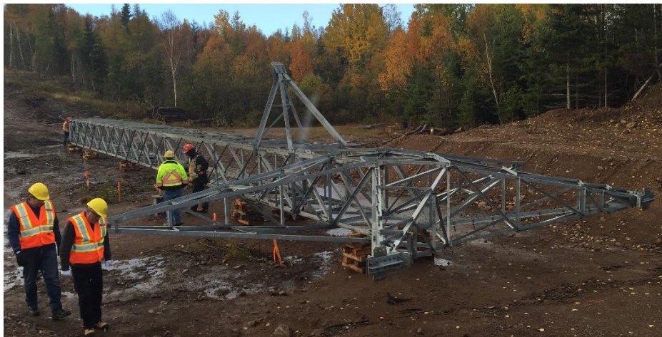
Photos 22, 23 & 24 - Cape Breton HVDC line – assembled guyed tower on ground ready for installation on pedestal foundation at left. Recently installed freestanding tower in centre background.
