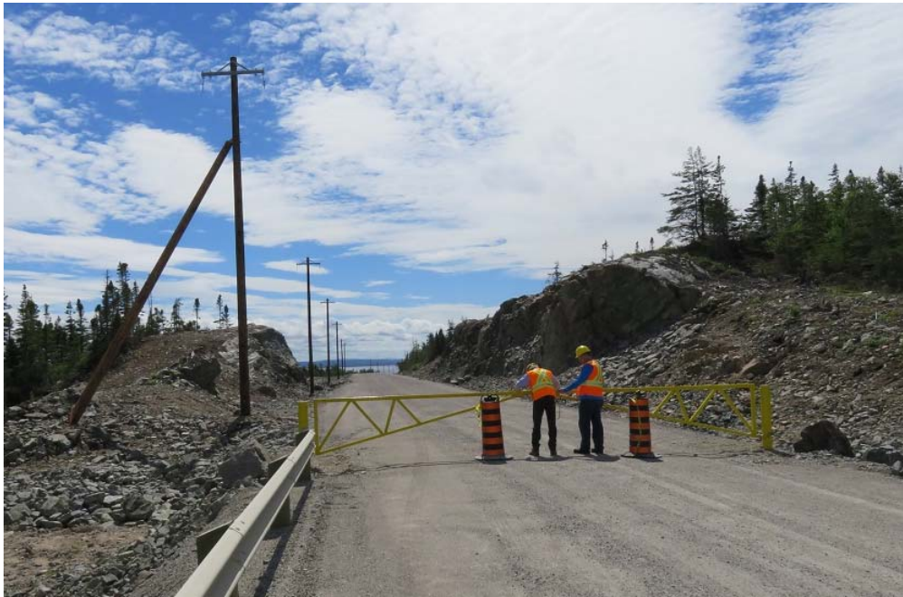
Photo 2 - Indian Head Grounding Site – View along completed site access road towards security gate and Indian Head site. Grounding lines have not yet been strung along this section of road. Showing an angle pole with a stub.
