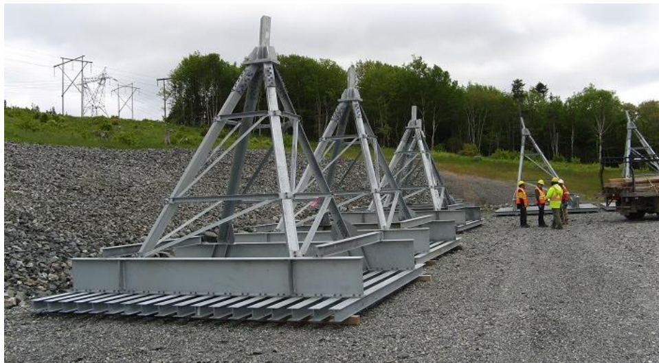
Photo 22 - Assembled type 2 grillages for tower 164 foundation. Rock covered slope in background is typical of permanent erosion protection along roads and ditches.
