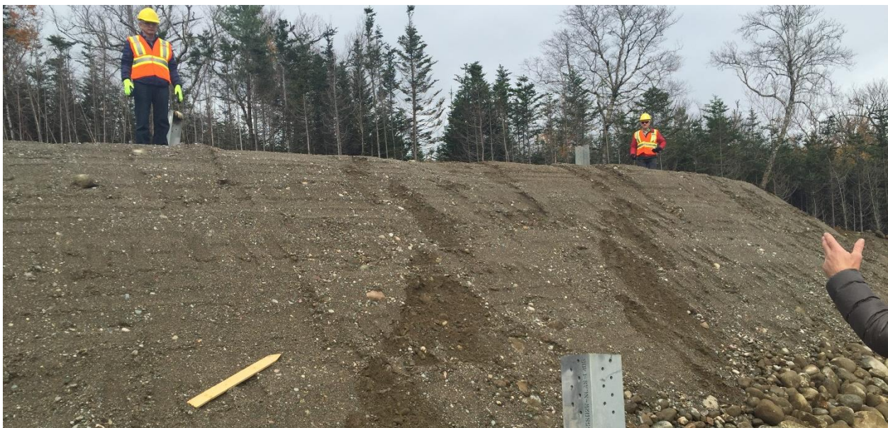
Photos 12 & 13 - HVDC line – steel tower footings installed on sloping ground at site SA7.
