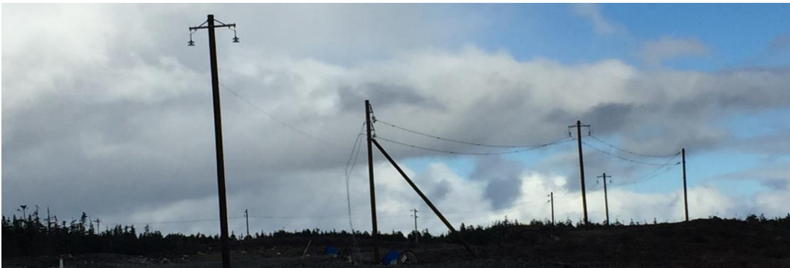
Photos 35 & 36 - Big Lorraine grounding site – end of the completed grounding line, awaiting completion of grounding site.
