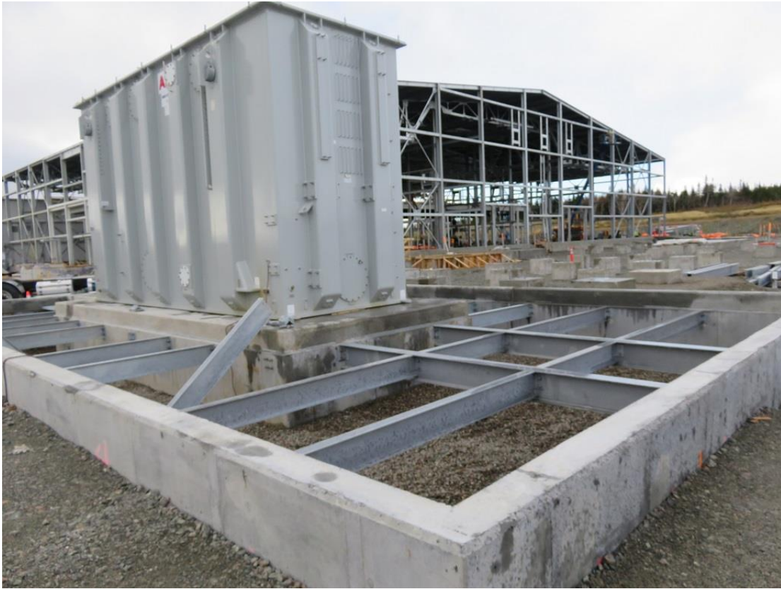
Photo 33 - Woodbine – ABB transformer installed on cast-in-place concrete foundation, with surrounding gravel-filled oil spill containment pit.
