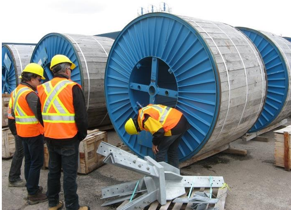
Photo 15 - DC conductor spools.
