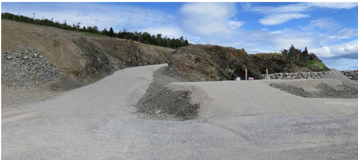
Photo 5 - Indian Head Grounding Site – View looking up access road at left. Overhead lines will terminate at pad at centre right side of photo.
