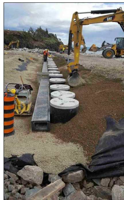
Grounding Wells at Indian Head
