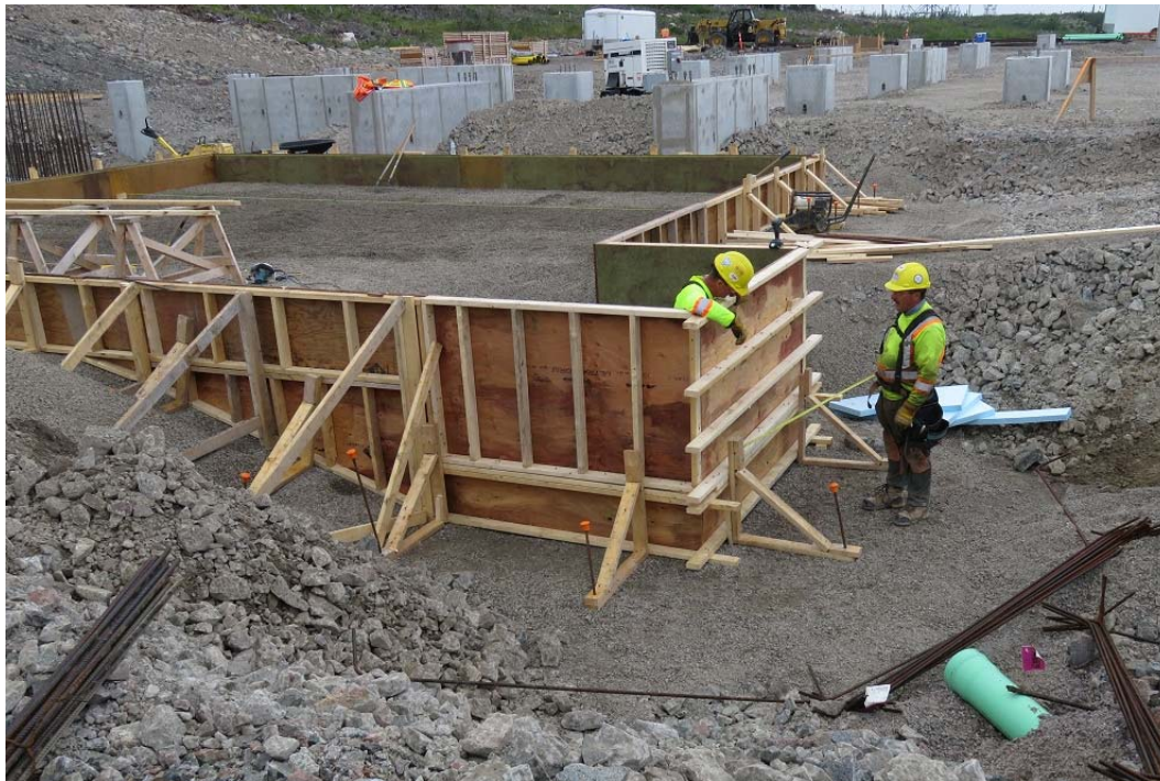
Photo 31 - Granite Canal Switchyard – Construction of formwork for concrete foundation for shunt reactor equipment.
