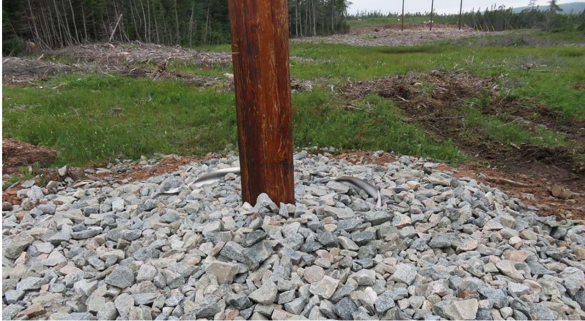
Photo 21 - HVAC line near Granite Canal – typical wood pole foundation in boggy ground; pole is installed inside a vertical section of corrugated metal pipe (culvert) which is then backfilled with crushed rock.
