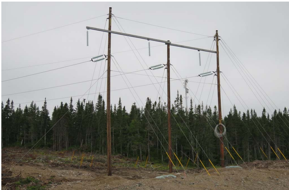
Photo 32 - HVAC line dead-end terminal structure adjacent to the Granite Canal switchyard. One side strung and the other side will be connected to the gantry structure in the switchyard.
