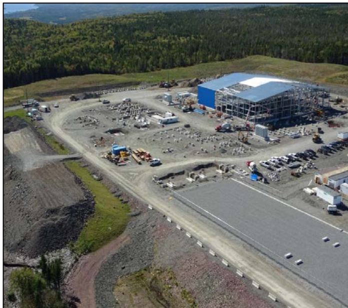
Converter building at Woodbine, NS, substation as of October, 2016
