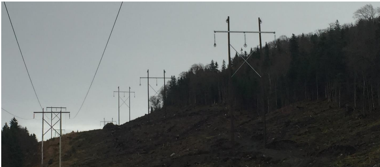
Photo 17 - HVAC – Easterly view looking beyond STR 259. New HVAC line at the right and existing line at left. Structure installation complete and waiting for the stringing.
