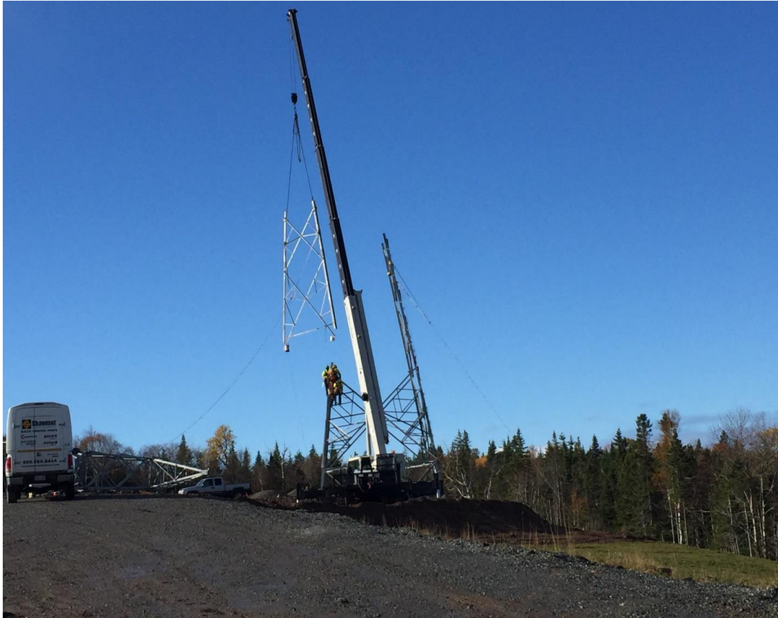
Photo 27 - Cape Breton HVDC line – tower erection in progress adjacent to Woodbine converter station site.
