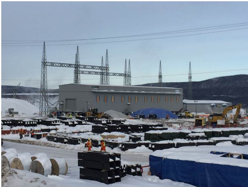
GIS and control building for the HVac substation at the Muskrat Falls transmission site
