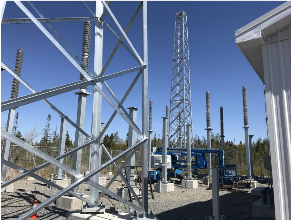
Photo 45: Transition compound control building, main gantry and post insulators.
