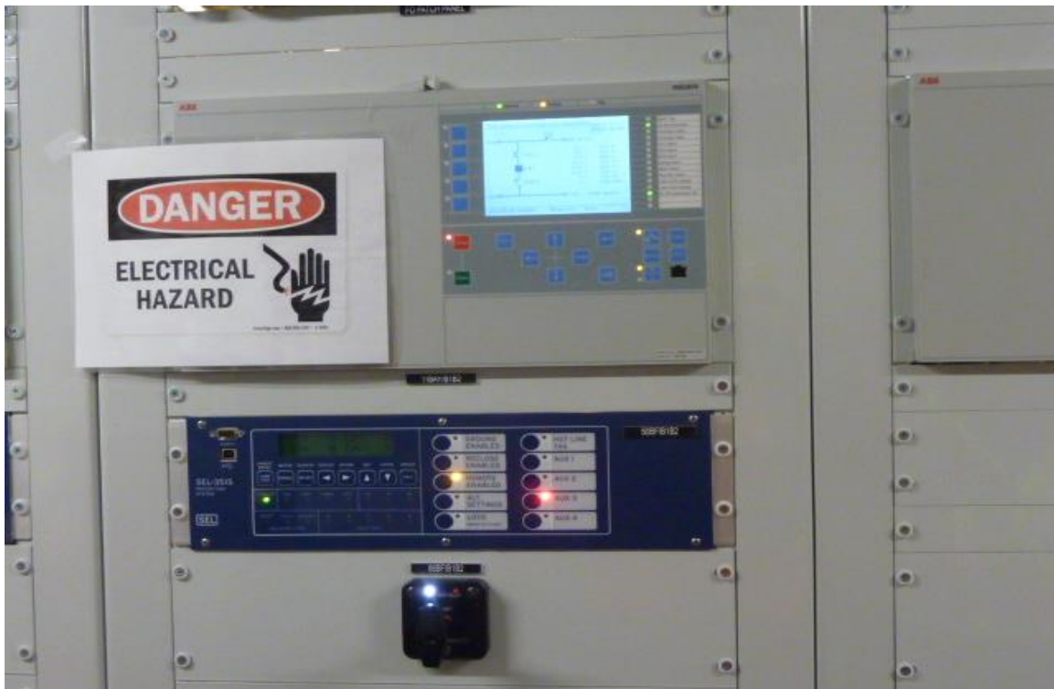
Photo 24: Diverse relay hardware from ABB and Schweitzer Engineering Ltd is employed in HVAC protection system.
