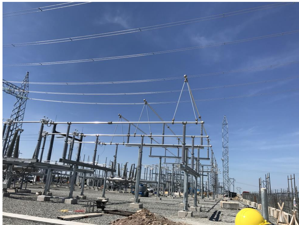
Photos 53: AC Substation yard.
