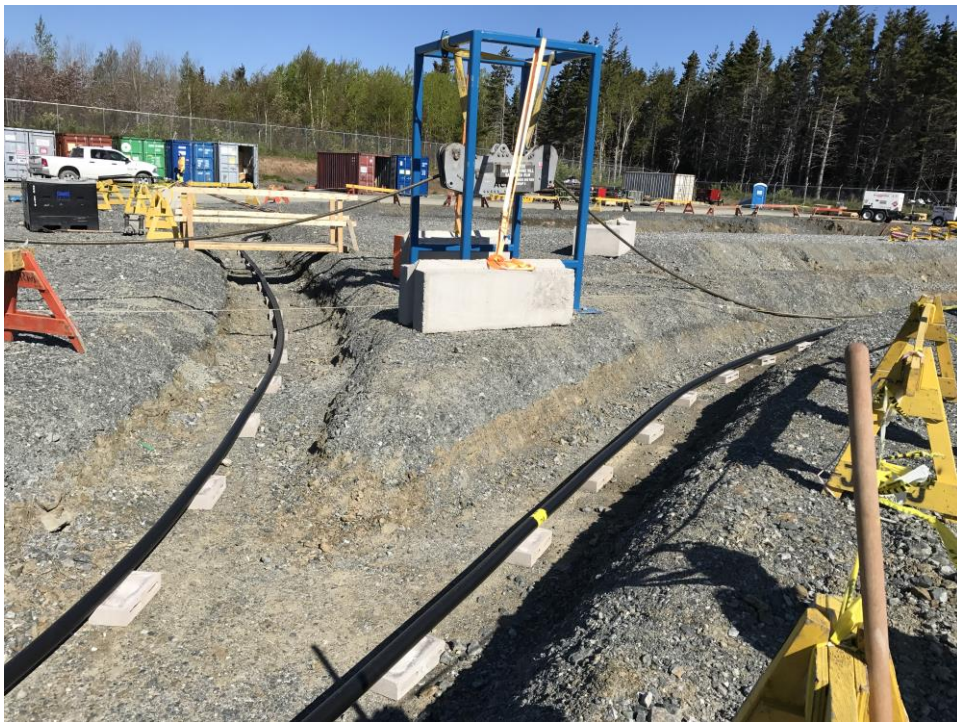
Photo 41: Land cables in trenches entering landfall site for jointing to subsea cables.
