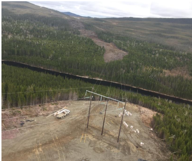
Photo 5. Corner dead end structure / AC line.
