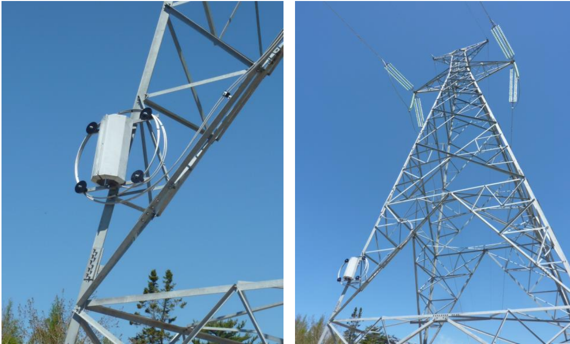
Photos 21/22: HVDC line fibreoptic box.
