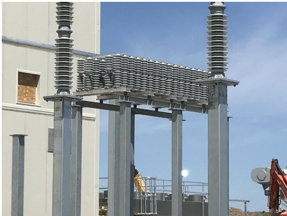
Photo 47: Close-up of surge arresters bank at the AC yard as part of the neutral bus.
