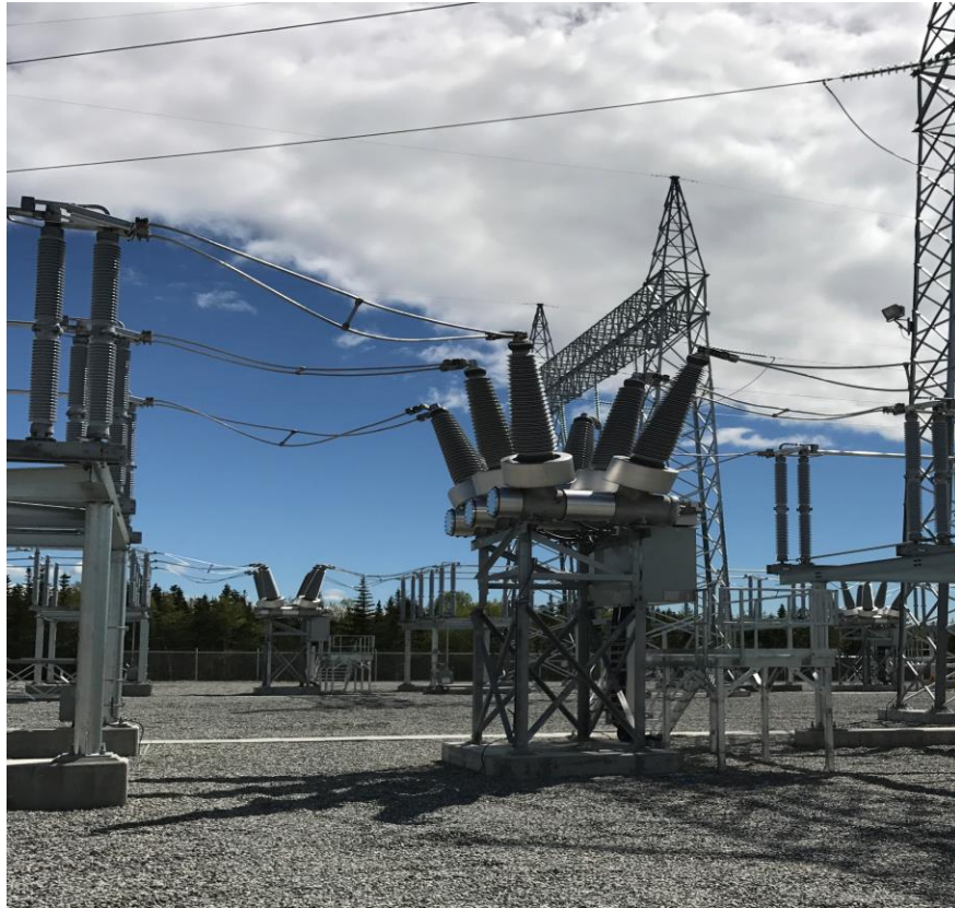
Photo 32: AC Substation - main 230 kV lines' circuit breakers.
