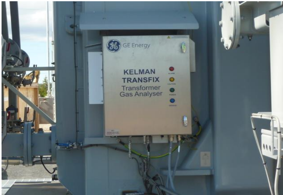
Photo 37: Converter transformer gas analyzer.
