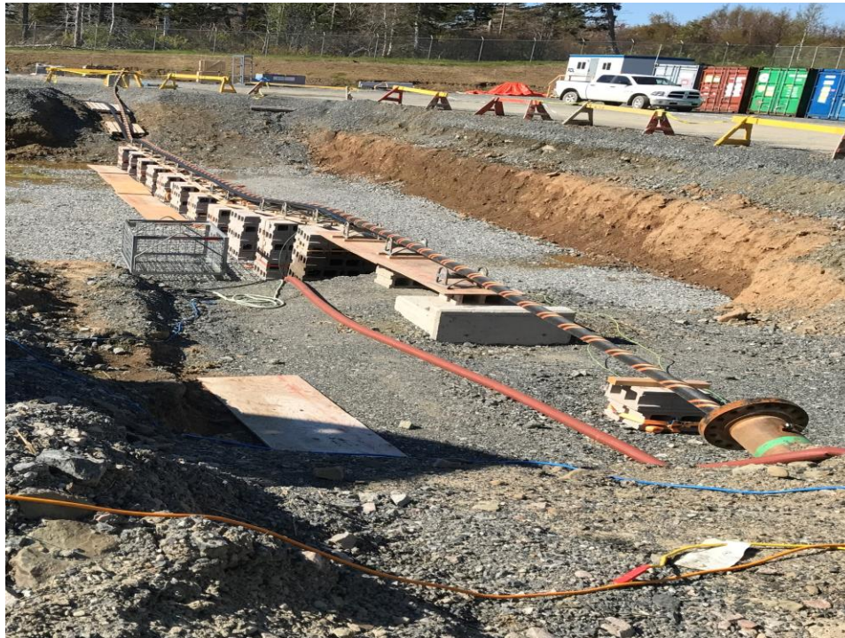
Photo 38: Cable 2 (West) already pulled in and in position for jointing with the land cable.
