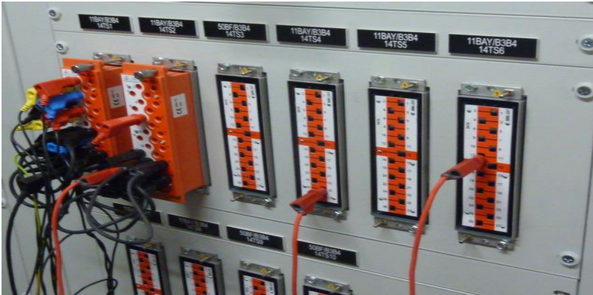
Photo 23. Details of Alstom test blocks and test lead connections.
