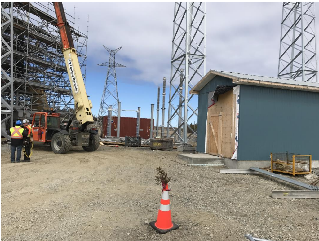
Photo 30: Transition compound control building, main gantry and post insulators.
