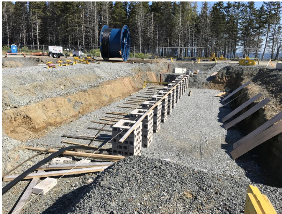
Photo 39: Site prepared for Cable 1 (East) pull - in. Land cable in position for jointing.
