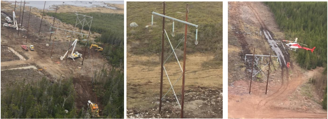
Photos 2/3/4. Stringing site / AC line – Structure ready for Stringing - Stringing using helicopter.
