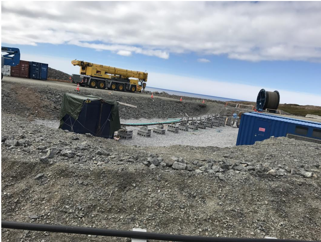
Photo 26: Subsea Cable 1 (east) already pulled through the HDD casing and ready for jointing.
