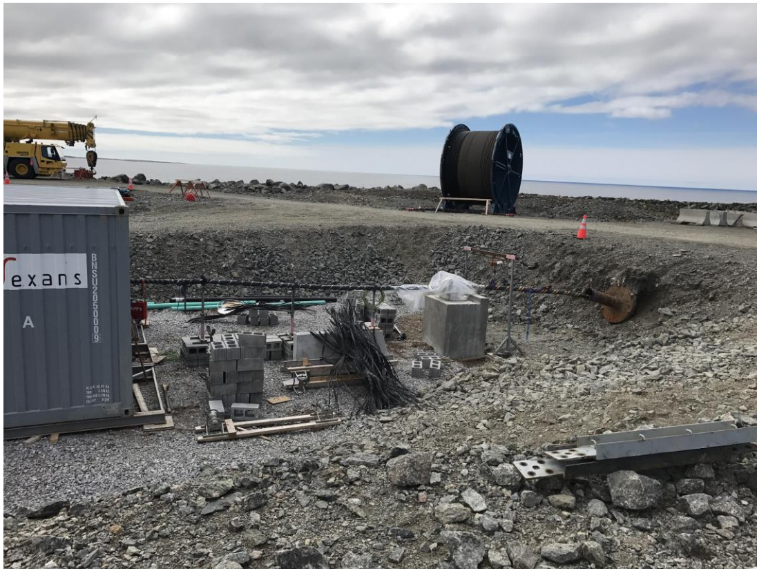
Photo 25: Subsea Cable 2 (west) already pulled through the HDD casing, anchored and in process of jointing to the land cable.
