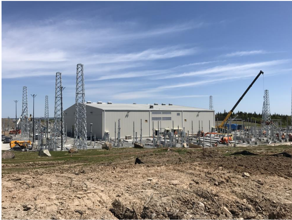
Photo 46: Converter Station building with the AC yard and part of the DC yard to the left.
