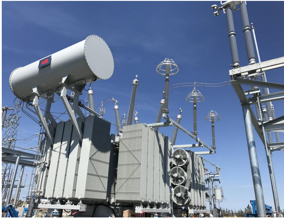
Photos 54: AC Substation autotransformer.
