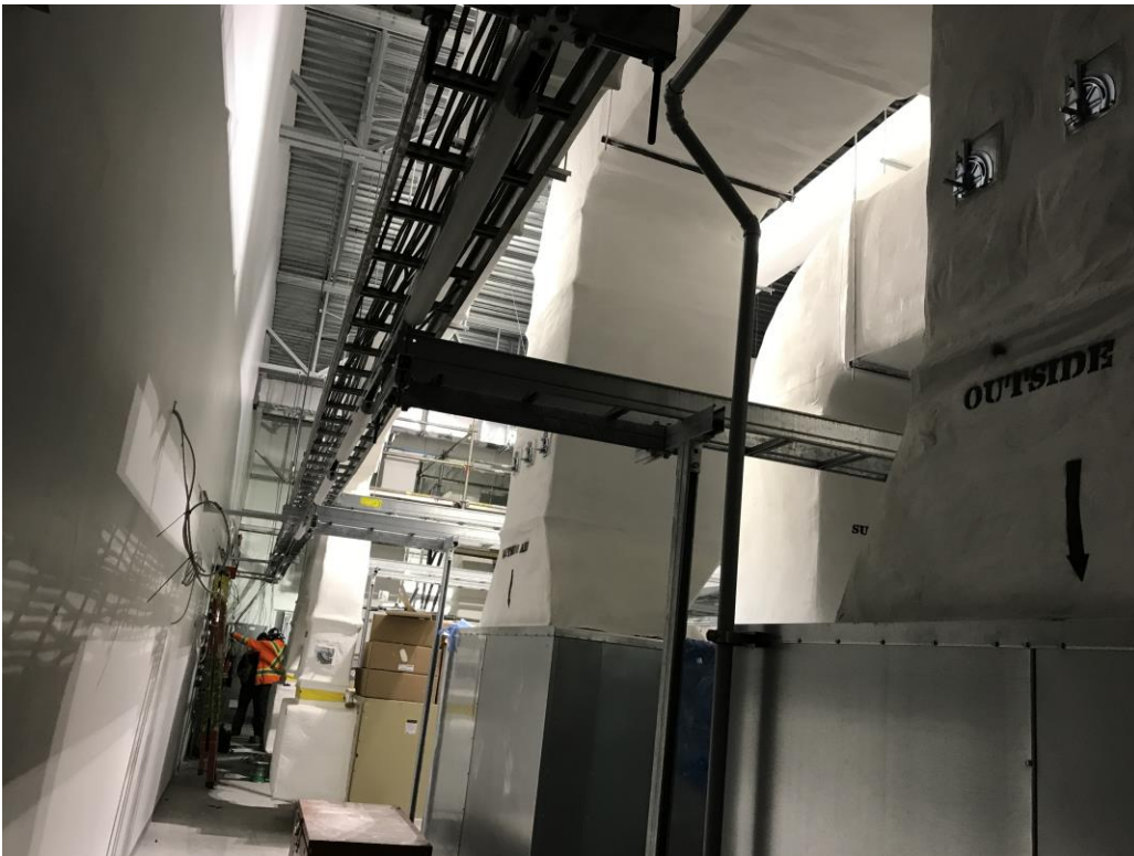
Photo 36: Converter Station – HVAC equipment installed on mezzanine level.
