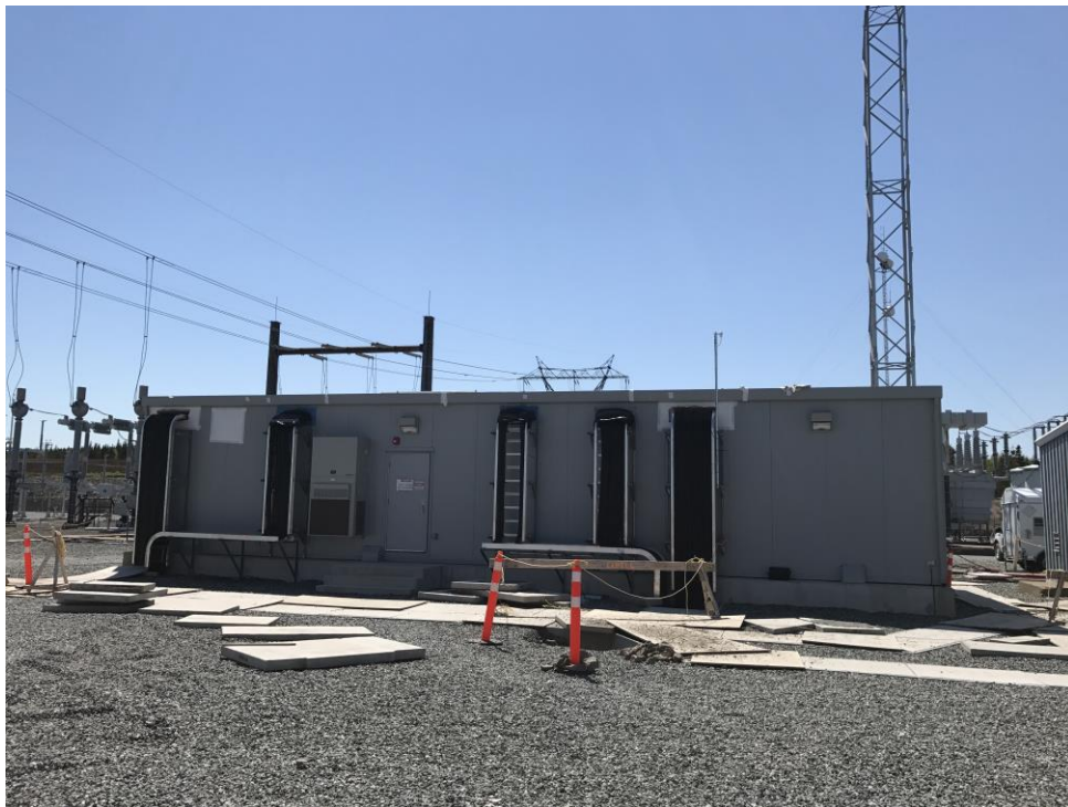
Photos 55: AC Substation control building.
