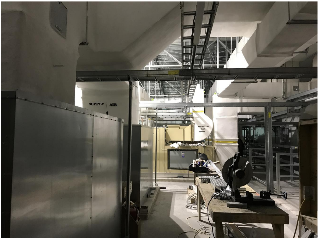
Photo 50: Converter Station – HVAC equipment installed on mezzanine level.
