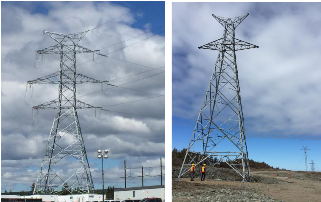
Photos 12/13. Double Circuit dead end tower / Single circuit self-supporting tower.
