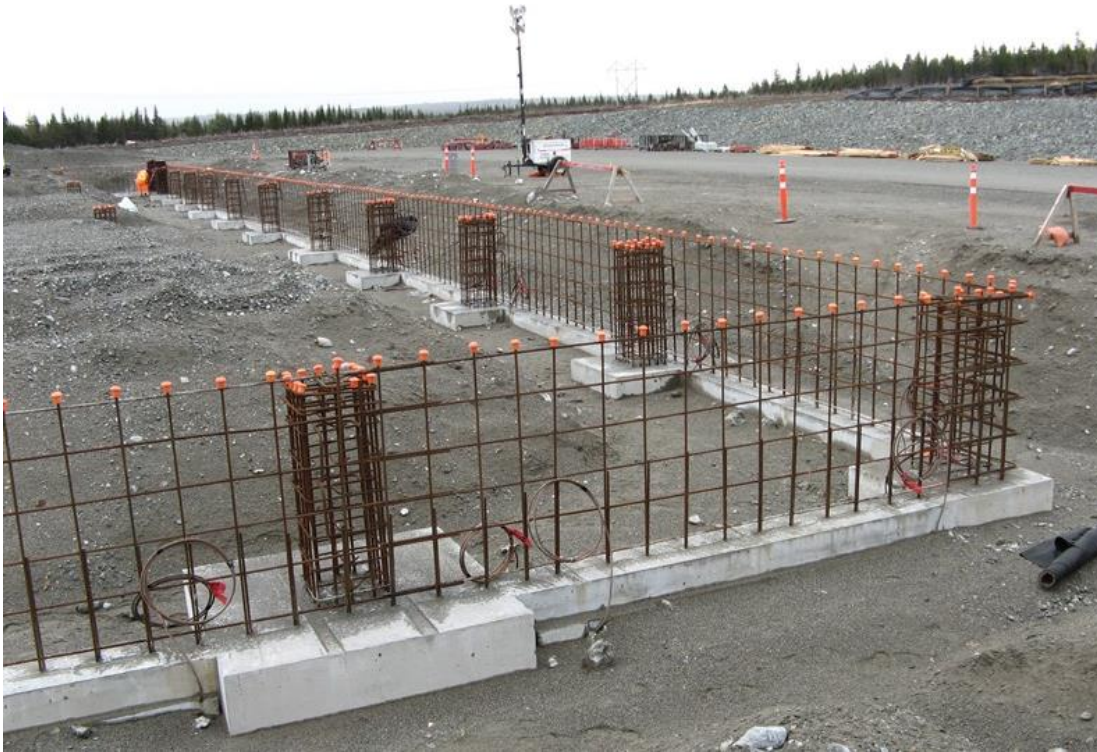
Photo 23: Bottom Brook – rebar for foundation wall of converter building in advance of installing concrete formwork.
