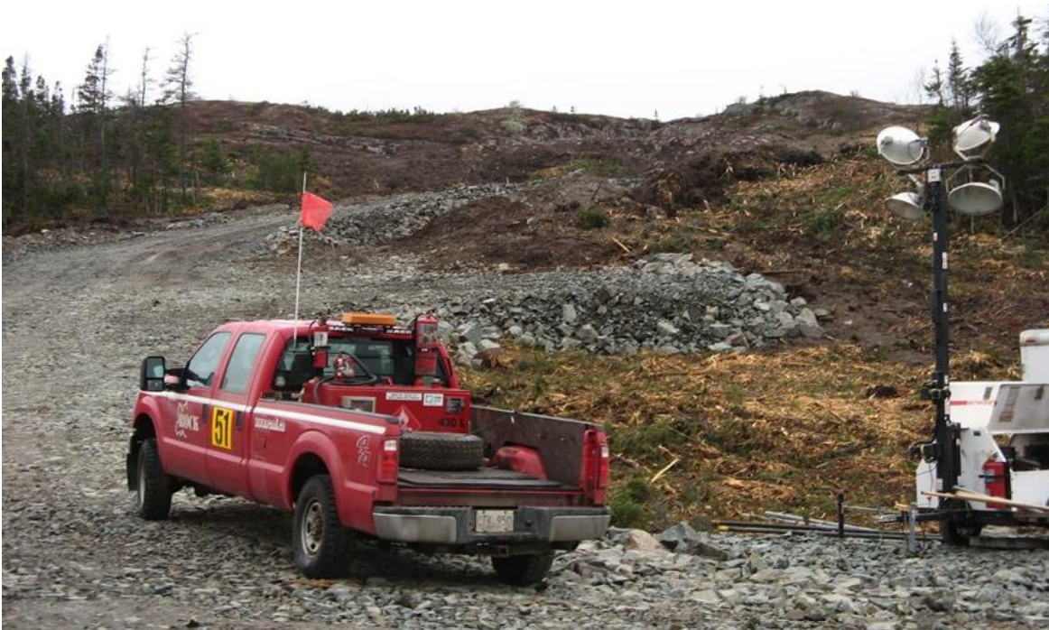
Photo 2: Indian Head – view from site access road looking up slope towards quarry site being developed to provide rockfill for construction of grounding station breakwater.
