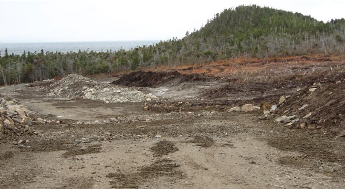
Photo 1: Indian Head - view looking down access road towards grounding site. Rockfill at left edge of photo is a safety berm along road. Rockfill berm at centre left will contain spoil material to be excavated from breakwater footprint.
