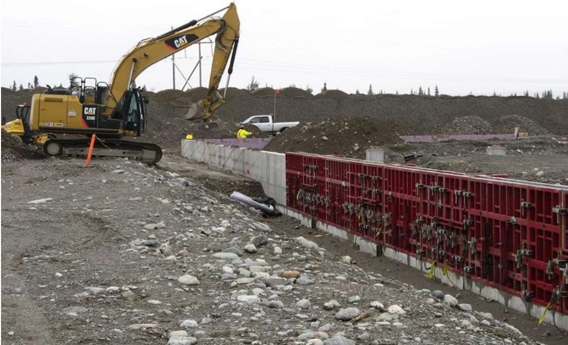
Photo 24: Bottom Brook – completed and recently-placed sections of concrete foundation wall of converter building.
