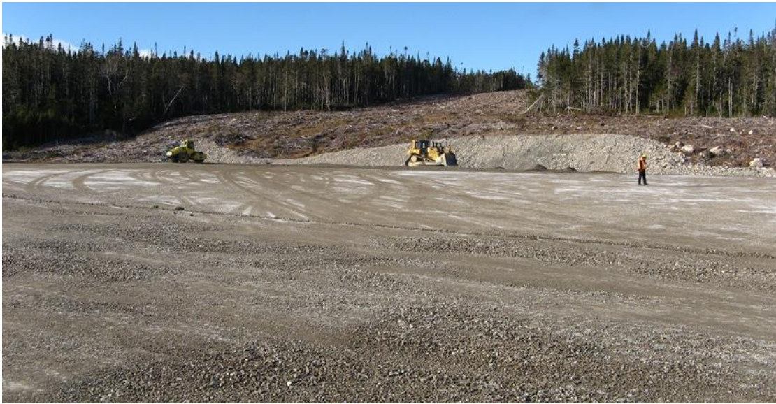
Photo 25: Granite Canalswitchyard – final construction of foundation pad in progress; east end of HVAC right-of-way in background.
