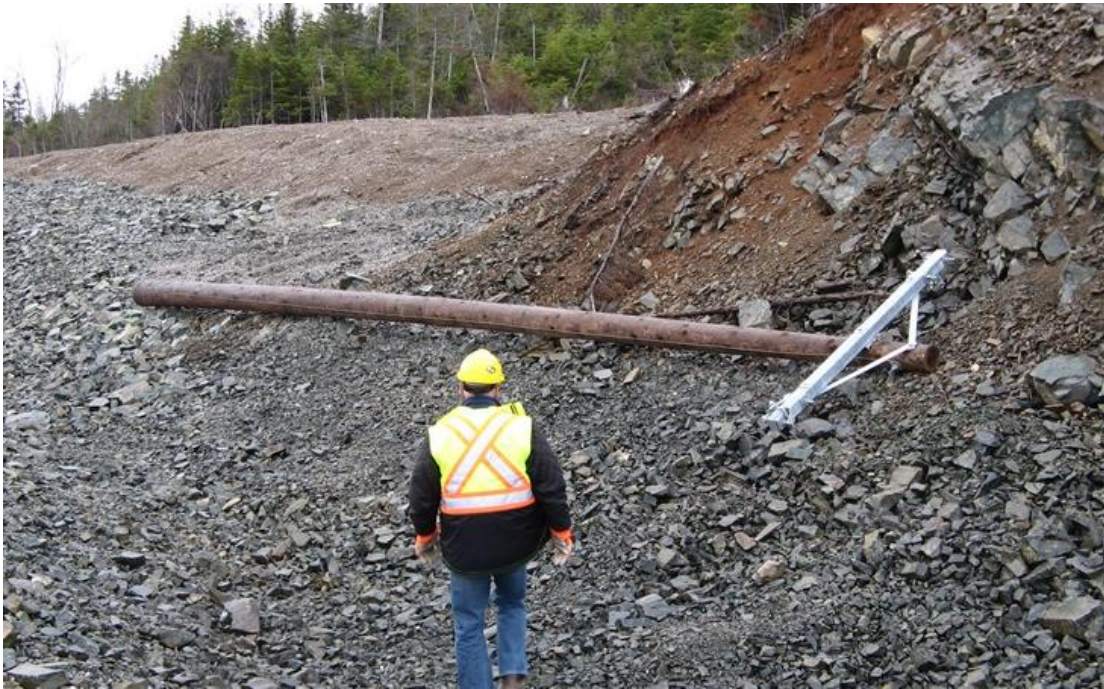
Photo 4: Indian Head – grounding line wood pole with galvanized steel crossarm, ready for installation.
