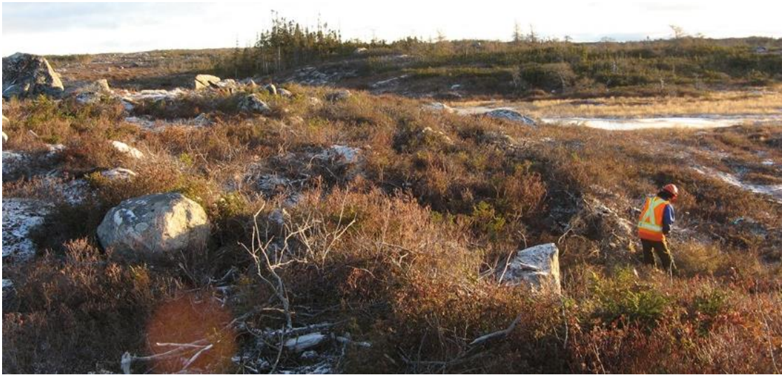
Photo 21: View looking easterly towards Granite Canal along HVAC right-of-way. Man at right is clearing brush with handheld power brush cutter.
