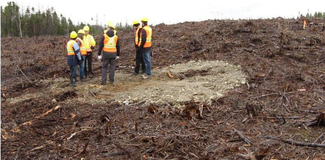
Photo 18: HVDC right-of-way adjacent to existing HVAC line. Wood debris has been shredded and scattered. Infilled test pit in centre of photo.
