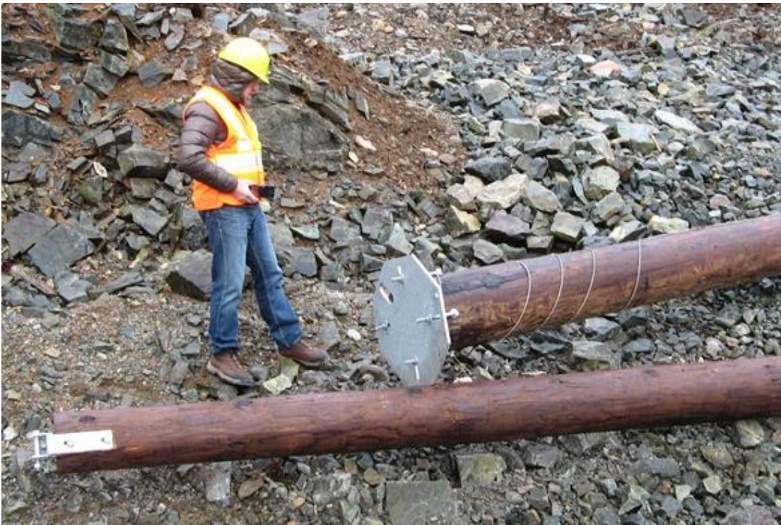
Photo 5: Indian Head – grounding line wood pole with galvanized steel base plate.
