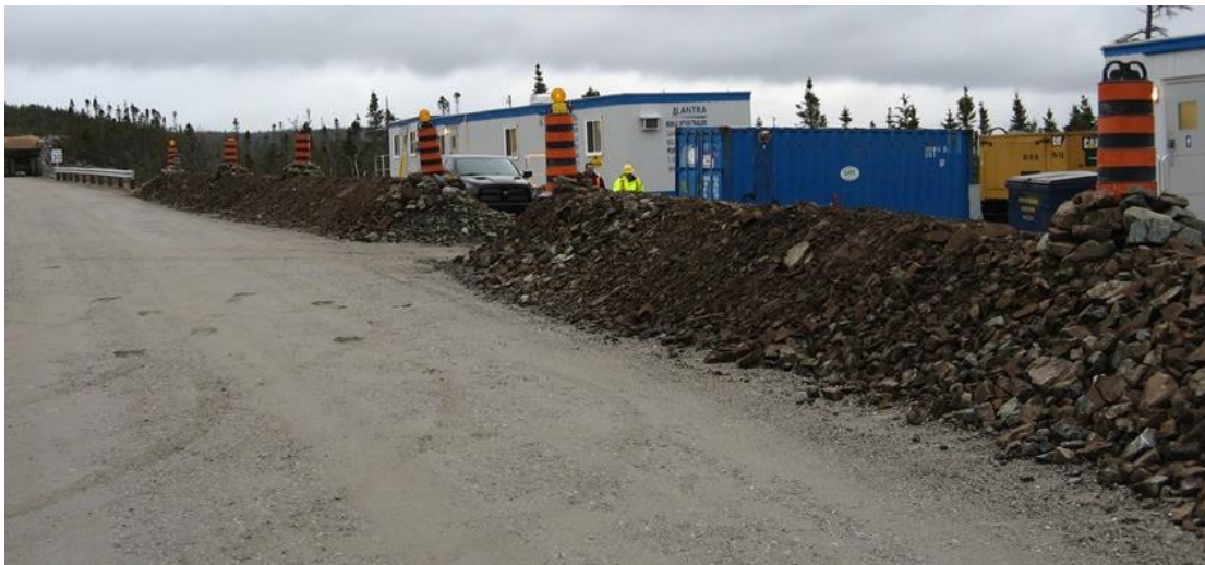
Photo 3: Indian Head – view looking along access road towards quarry, showing safety berm constructed between access road and contractor facilities.
