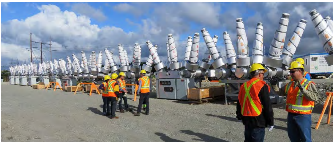
Photo 17 - Bottom Brook – Circuit breakers supplied by ABB, awaiting installation.
