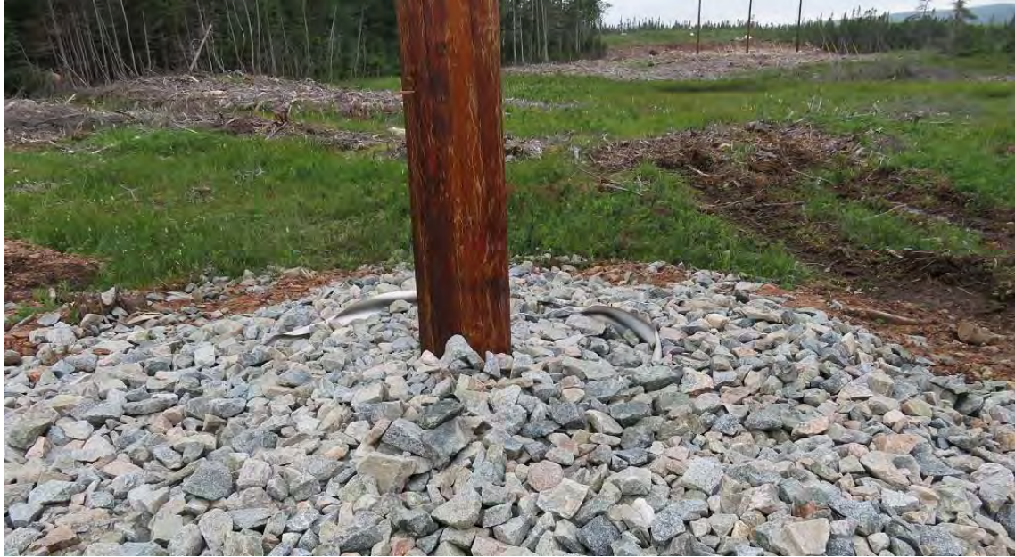
Photo 21 - HVAC line near Granite Canal – typical wood pole foundation in boggy ground; pole is installed inside a vertical section of corrugated metal pipe (culvert) which is then backfilled with crushed rock.
