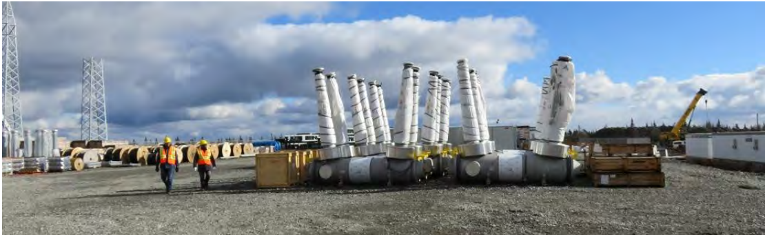
Photo 32 - Woodbine – ABB circuit breakers awaiting installation in switchyard. Spools of cable and other materials located at left side of photo.
