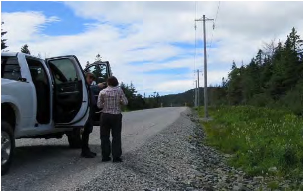
Photo 1 - Indian Head Grounding Site – View towards Indian Head site along completed site access road near Hwy. 490 turnoff. Grounding lines have been strung along this section of road.
