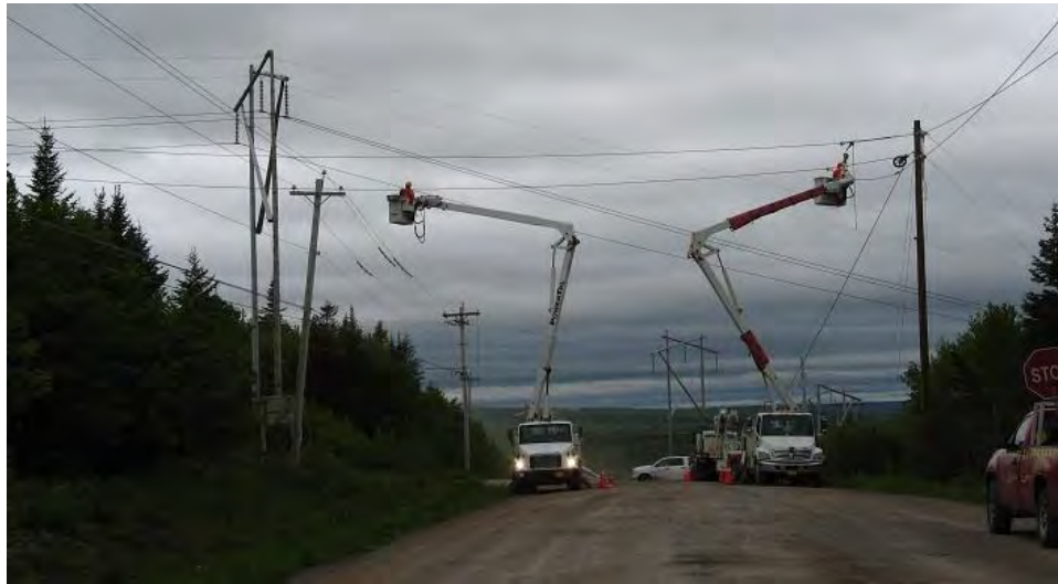
Photo 28 - Stringing grounding line across road near entrance to Woodbine converter station (PowerTel is contractor)
