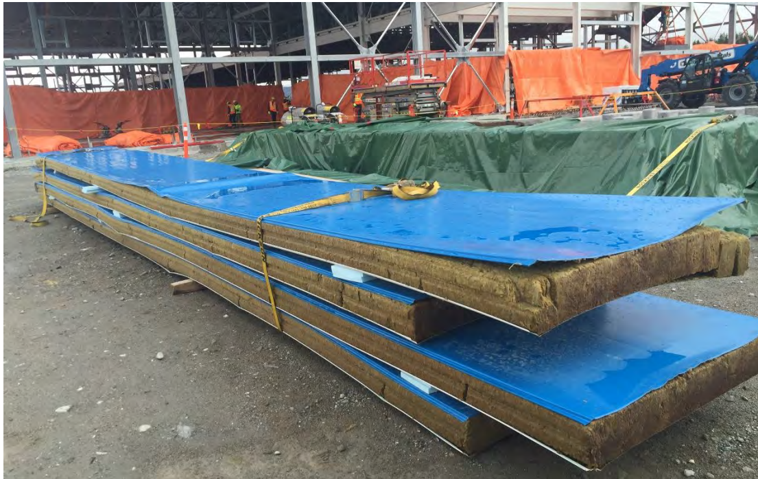
Photos 3 & 4 - Bottom Brook – buckling of insulated wall cladding panel that occurred when initial installation was attempted.
