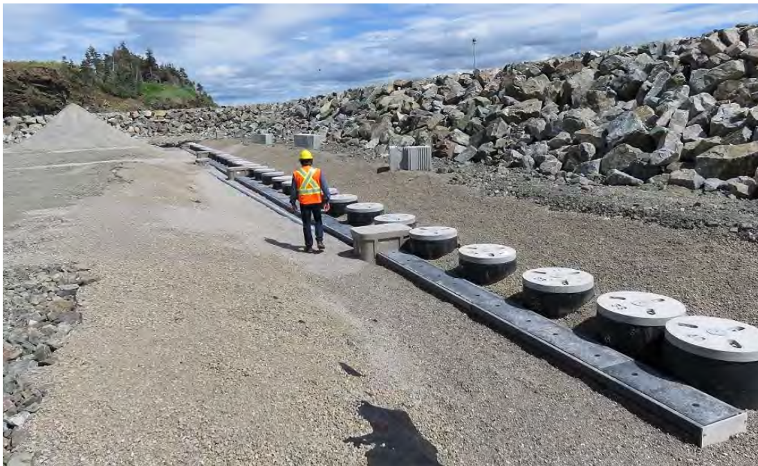
Photo 7 - Indian Head Grounding Site – View inside of rock berm (electro yard) showing row of 40 grounding wells awaiting installation of grounding electrodes, with adjacent cable duct.
