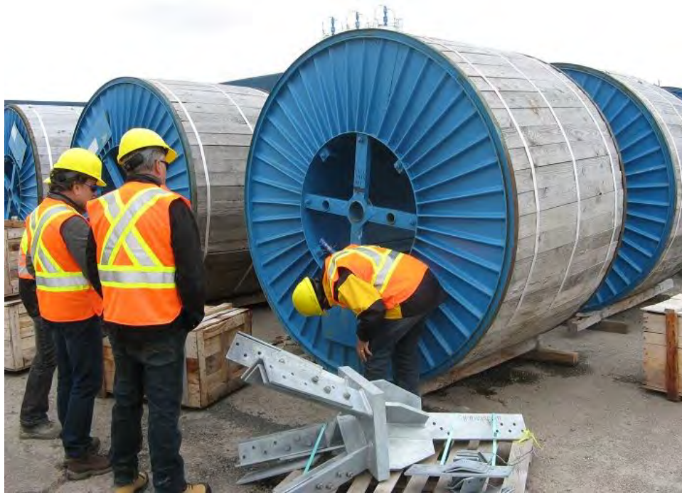
Photo 15 - DC conductor spools.
