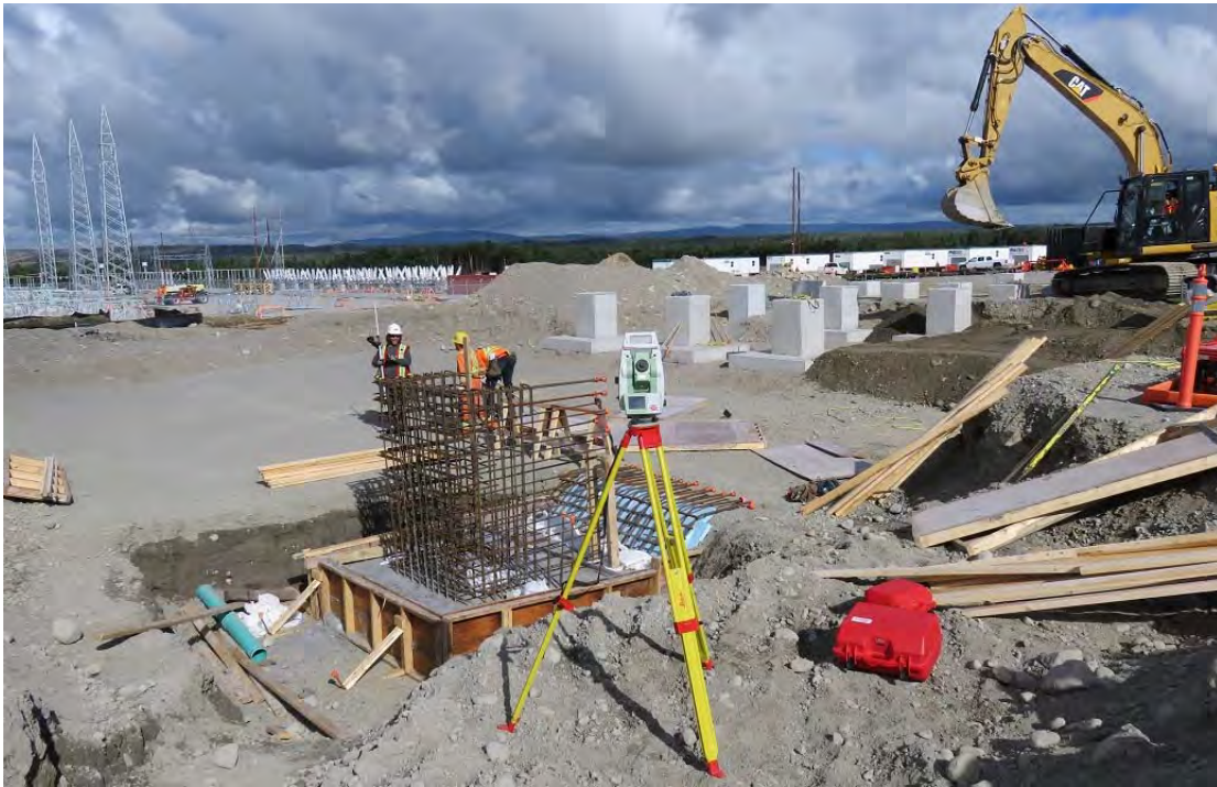
Photo 16 - Bottom Brook – General view of a cast-in-place concrete equipment footing in foreground, with closely-spaced precast concrete footings being installed in centre right of photo. Note the safetycaps on exposed horizontal rebar ends.
