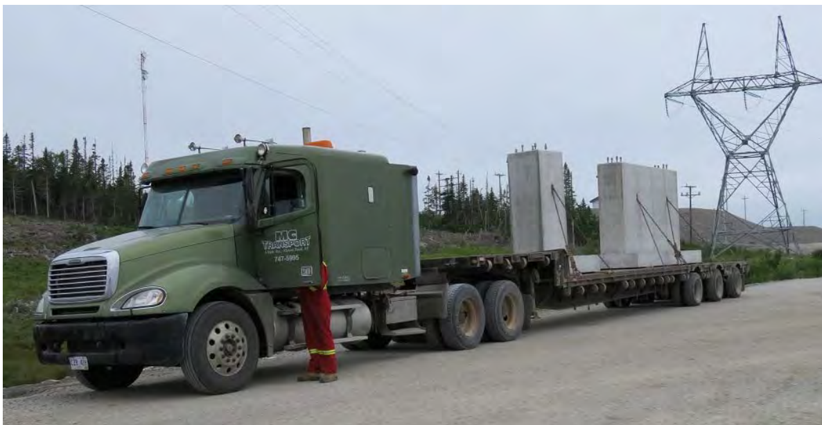
Photo 28 - Granite Canal Switchyard – two precast concrete footings being delivered from St. John's.
