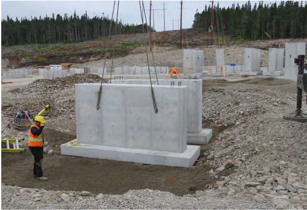
Photo 29 - Granite Canal Switchyard – mobile crane placing precast concrete footing on prepared sub-base.
