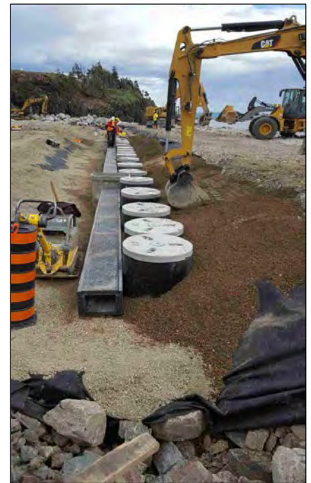
Grounding Wells at Indian Head
