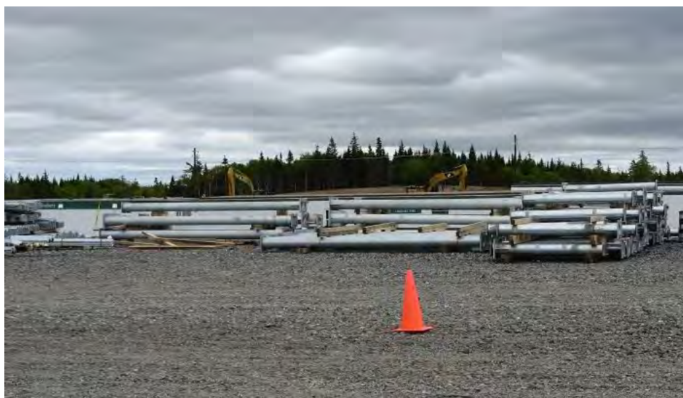
Photo 24 - Components for new DC switchyard.
