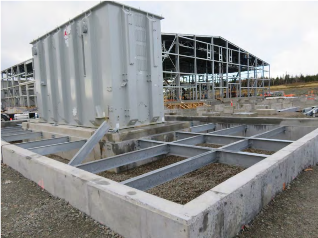
Photo 33 - Woodbine – ABB transformer installed on cast-in-place concrete foundation, with surrounding gravel-filled oil spill containment pit.
