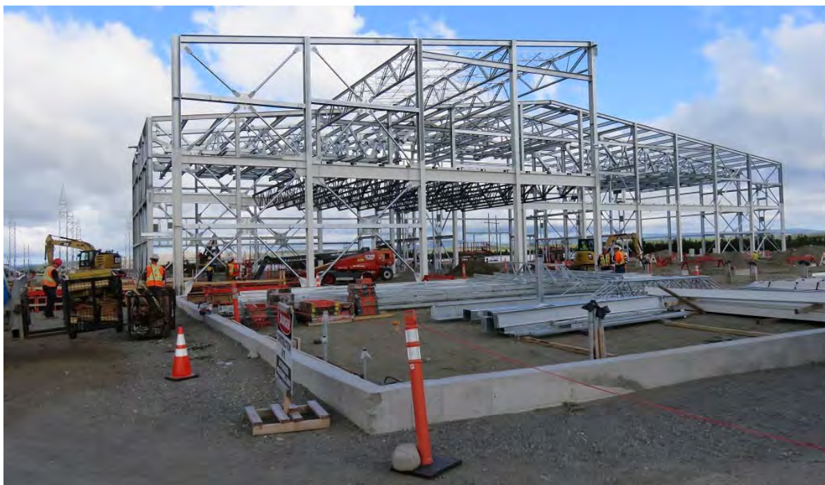
Photo 13 - Bottom Brook – partially-erected steel frame for converter building. The concrete foundation in foreground indicates the full extent of the building when it is completed.
