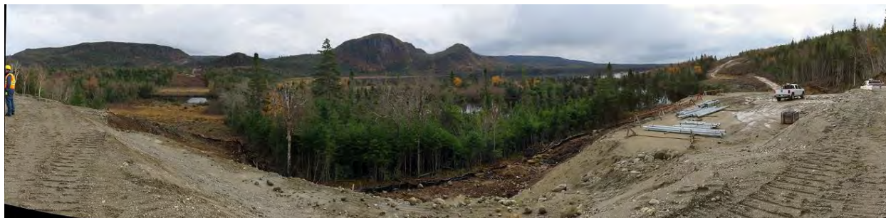
Photo 9 - HVDC line – panorama view of HVDC right of way from site SA7. Right-of-way crosses Bottom Brook at left. Steel for tower mobilized to site at right.
