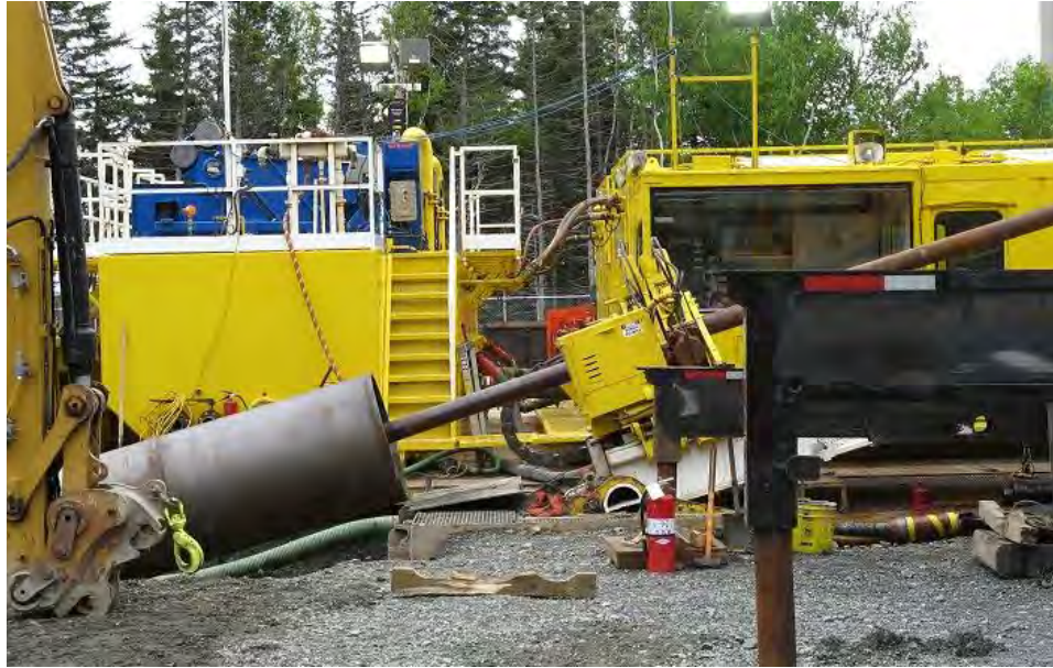
Photo 2 - Large 42-inch diameter pipe is a steel casing. Smaller pipe inside casing is the drill rod which connects to a 36-inch diameter auger bit being used to drill the pilot hole. Drill operator is located in glass booth at right side behind drill rig.
