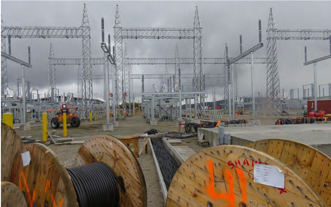
Photo 5 - Bottom Brook – general view of completed structural steel in substation with cable duct in foreground.
