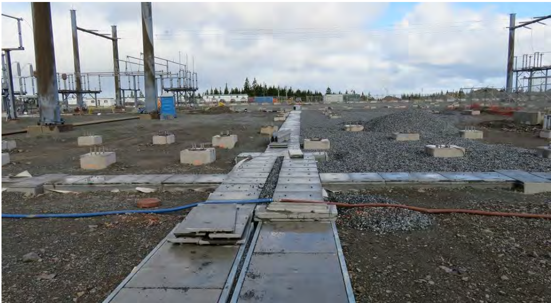
Photo 31 - Woodbine – view along cable ducts in AC substation , with numerous precast concrete footings installed and ready for structural steel and equipment installation.
