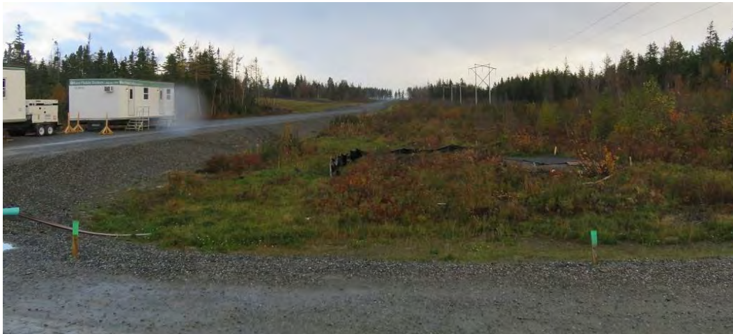
Photo 20 - View from transition compound site towards Point Aconi landfall. Underground HVDC cables will be installed along side of road.
