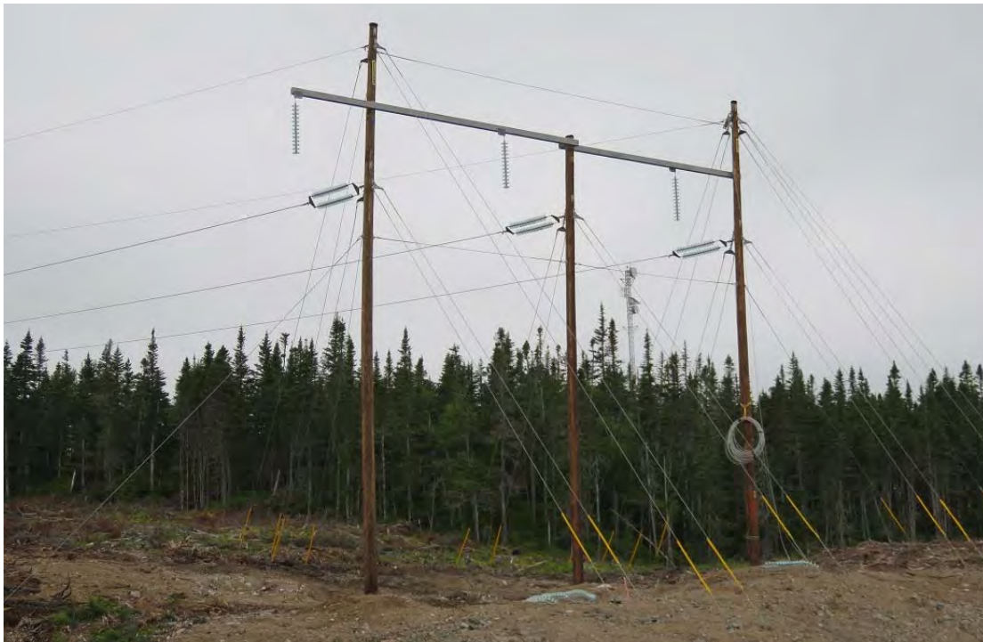
Photo 32 - HVAC line dead-end terminal structure adjacent to the Granite Canal switchyard. One side strung and the other side will be connected to the gantry structure in the switchyard.
