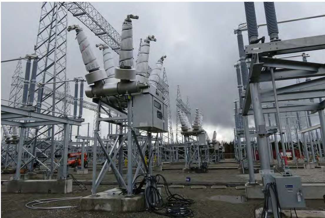
Photo 6 - Bottom Brook – ABB circuit breakers installed on concrete footings.
