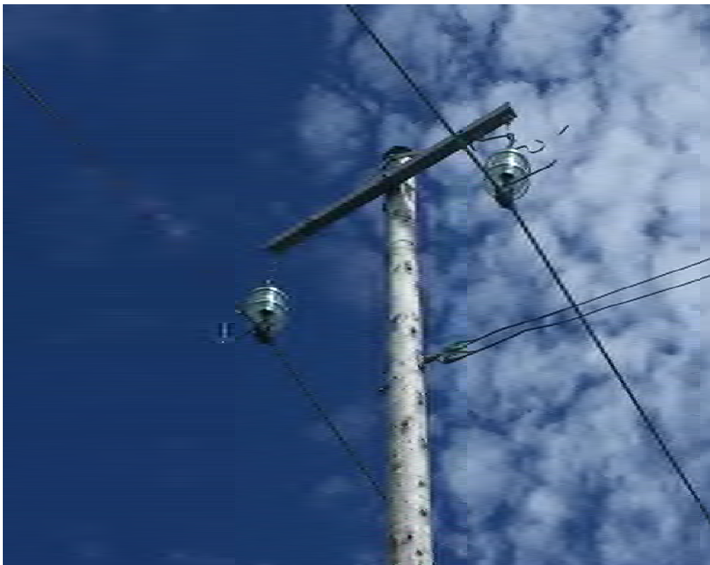
Photo 3 - Close picture for the strung grounding line – Sample tangent structure
