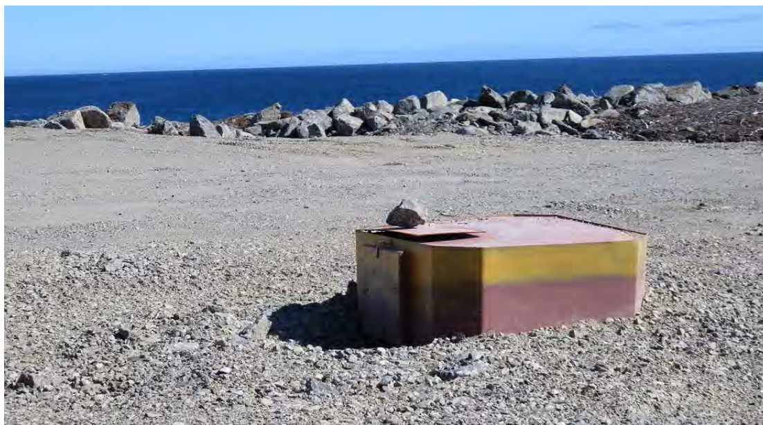
Photo 9 - Cape Ray landfall site – temporary protective cover on one of the two HDD hole collars.
