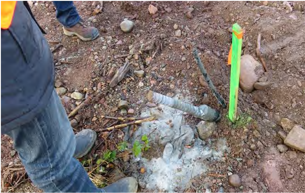
Photo 25 - Cape Breton HVDC line – typical grouted thread bar foundation anchor for guyed tower.
