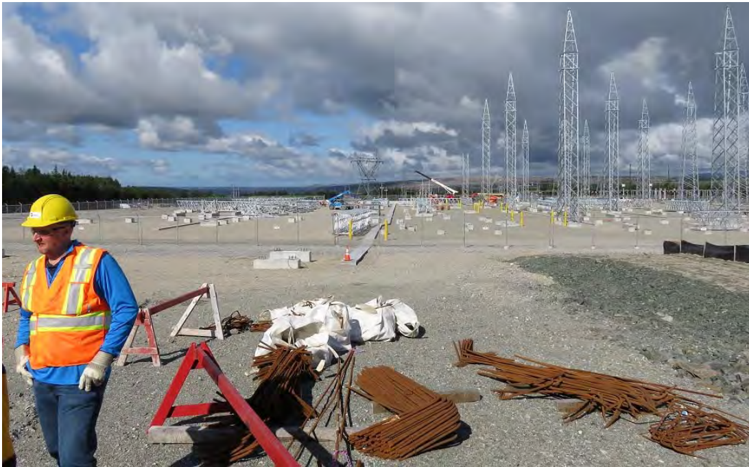
Photo 14 - Bottom Brook – switchyard construction in progress, with recently erected steel structures at right and other assembled structures laying on the ground awaiting erection at left.
