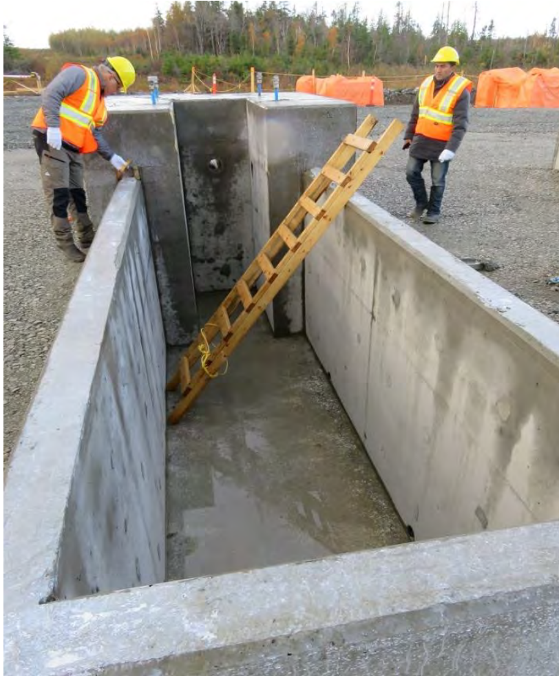
Photo 21 - Point Aconi transition compound – completed concrete vault with footing for termination structure. The HVDC land cable will transition in the vault from underground to overhead. Other concrete footings are covered by tarps in background.
