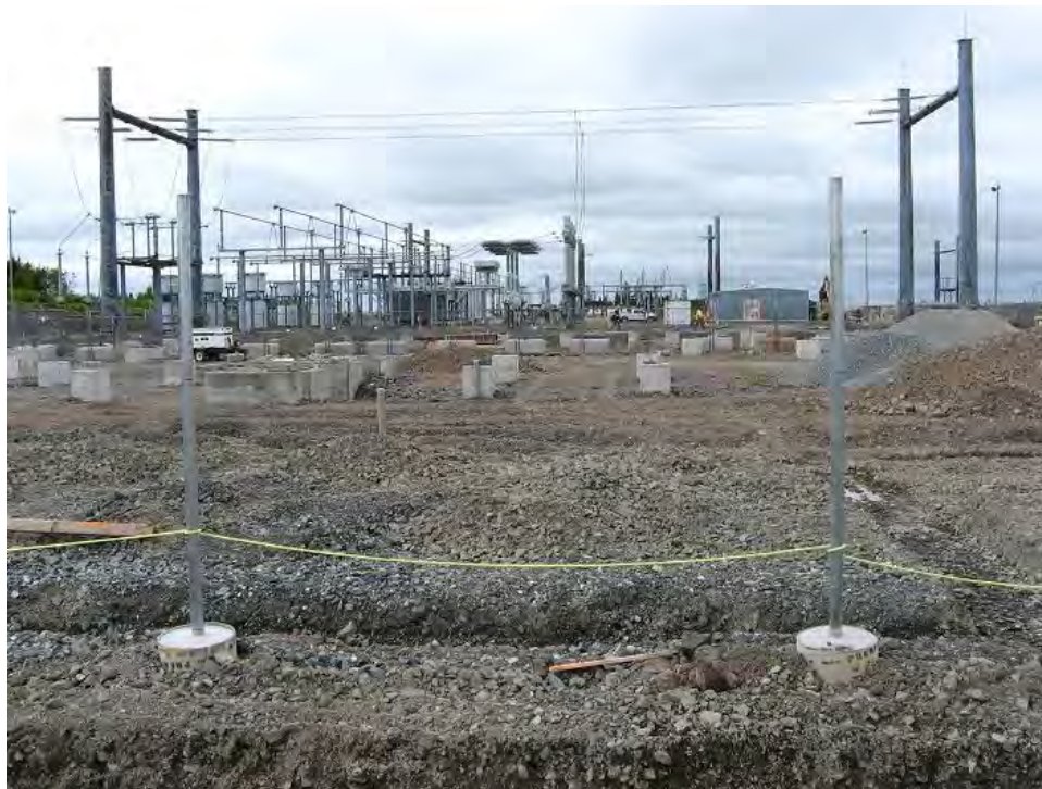
Photo 23 - Expansion of existing AC switchyard. Most of the concrete footings in foreground are precast.
