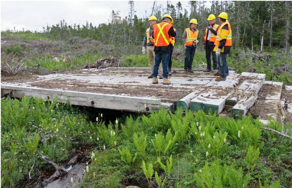
Photo 27 - HVAC line near Granite Canal – typical crossing of small watercourse using timber mats.
