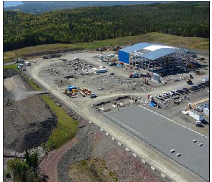
Converter building at Woodbine, NS, substation as of October, 2016
