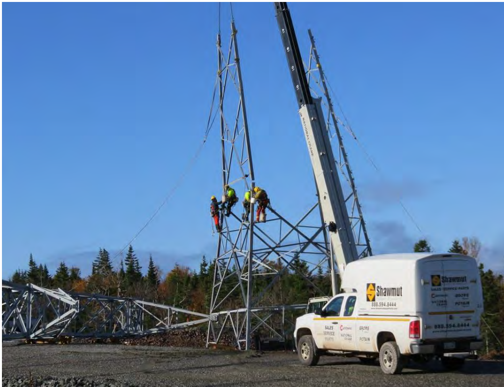
Photo 26 - Cape Breton HVDC line – tower erection in progress adjacent to Woodbine converter station site.
