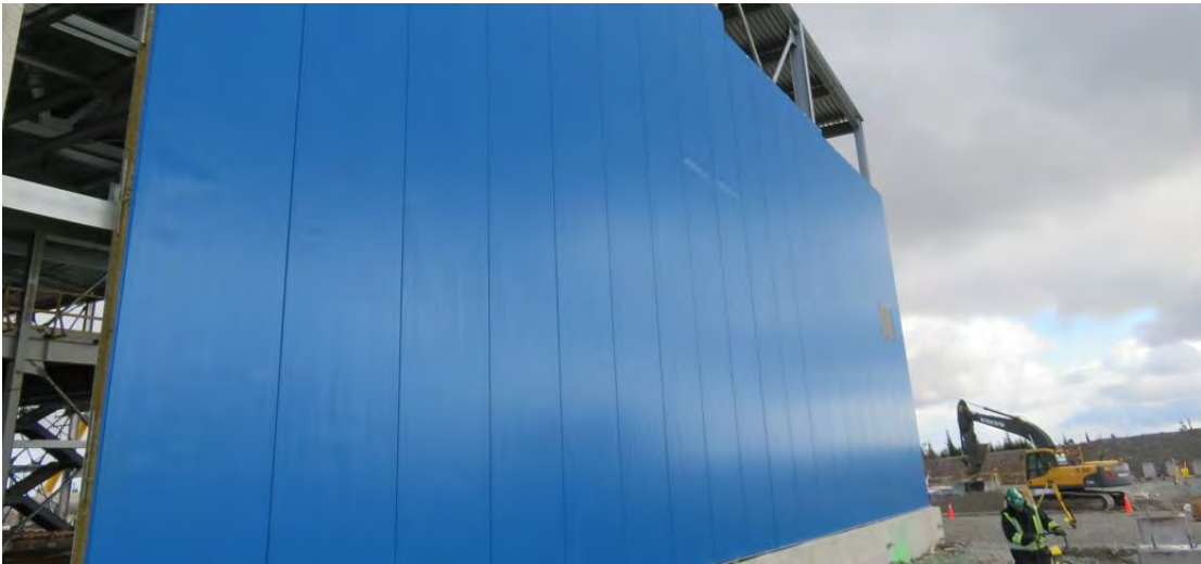
Photo 29 - Woodbine – close-up view of installed wall cladding showing several surficial buckled zones. This cladding was to be removed and replaced.
