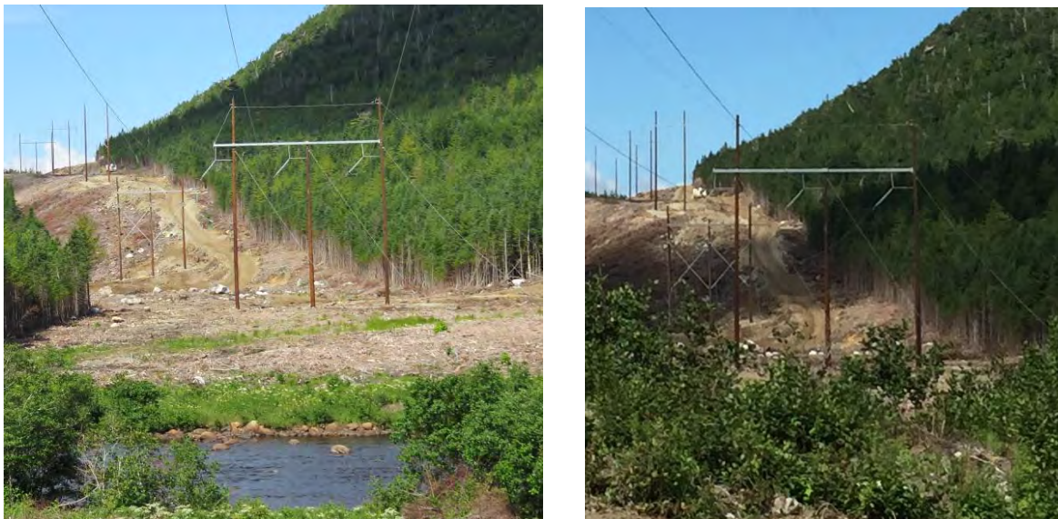
Photo 18 - HVAC line at crossing of Southwest Brook along Burgeo Highway, with three-pole angle structures in foreground and two-pole structures in background.
