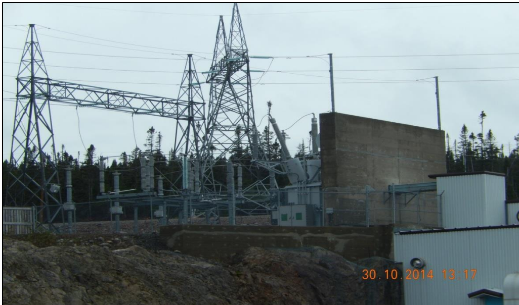
Existing Granite Canal Terminal Station
