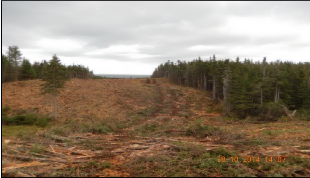
Land clearing for access road and grounding line ROW to the grounding site
