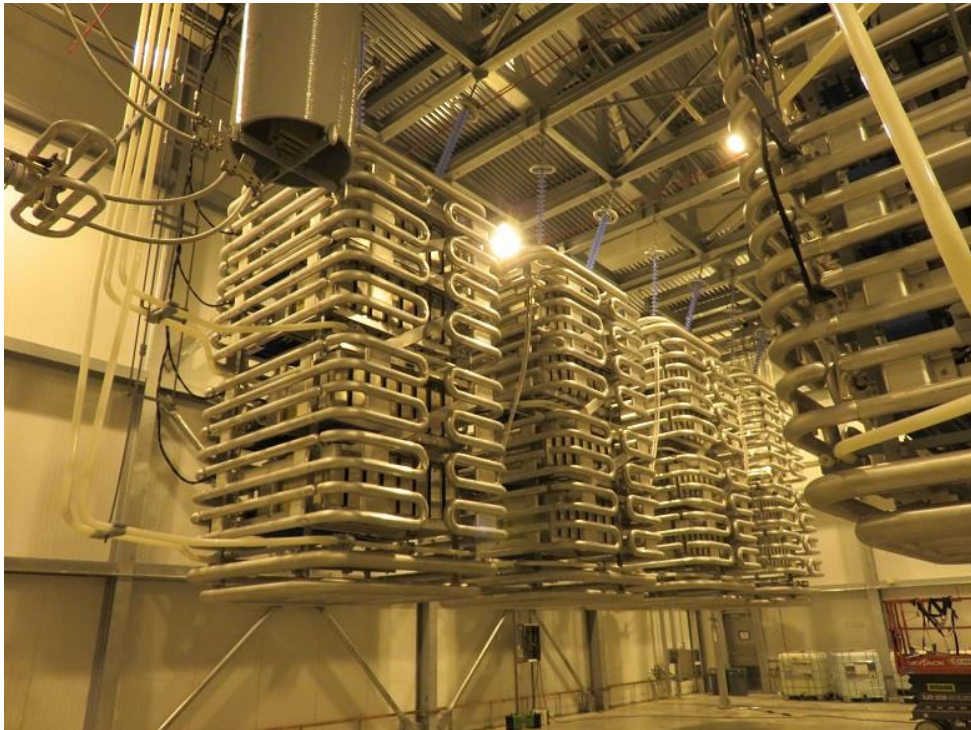
Photo 8: Pole 1 valve hall at Bottom Brook converter building.
