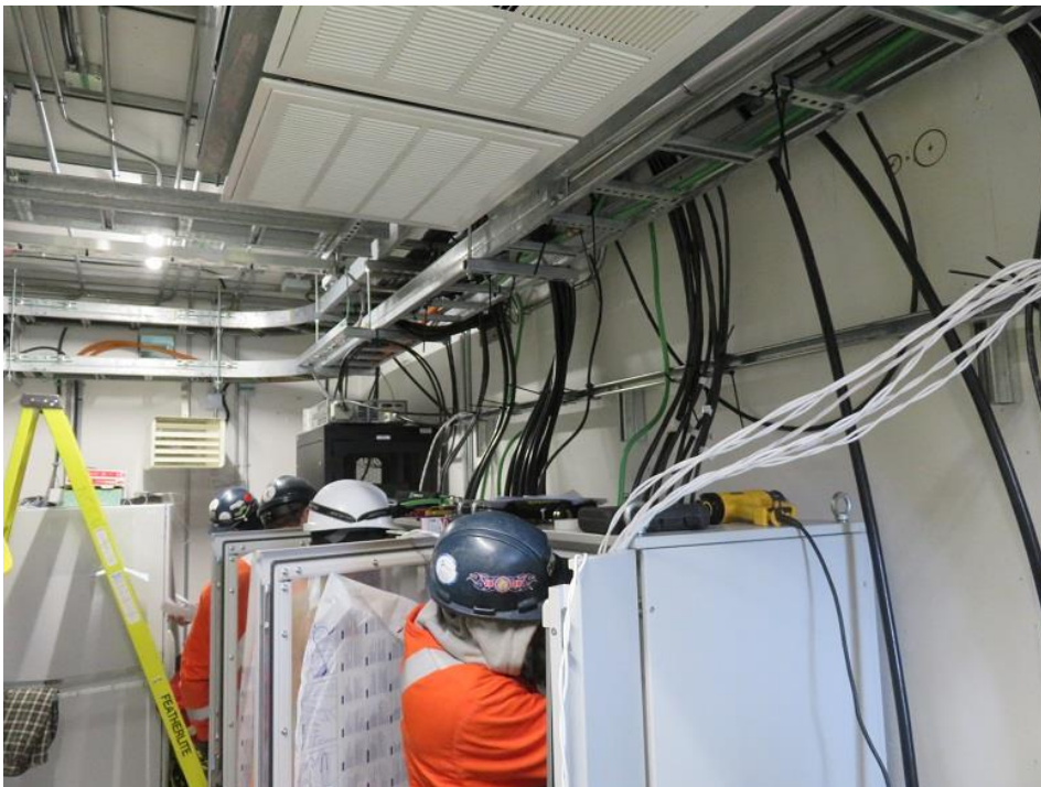
Photo16: Point Aconi transition compound - Control panel installation in progress inside service building.
