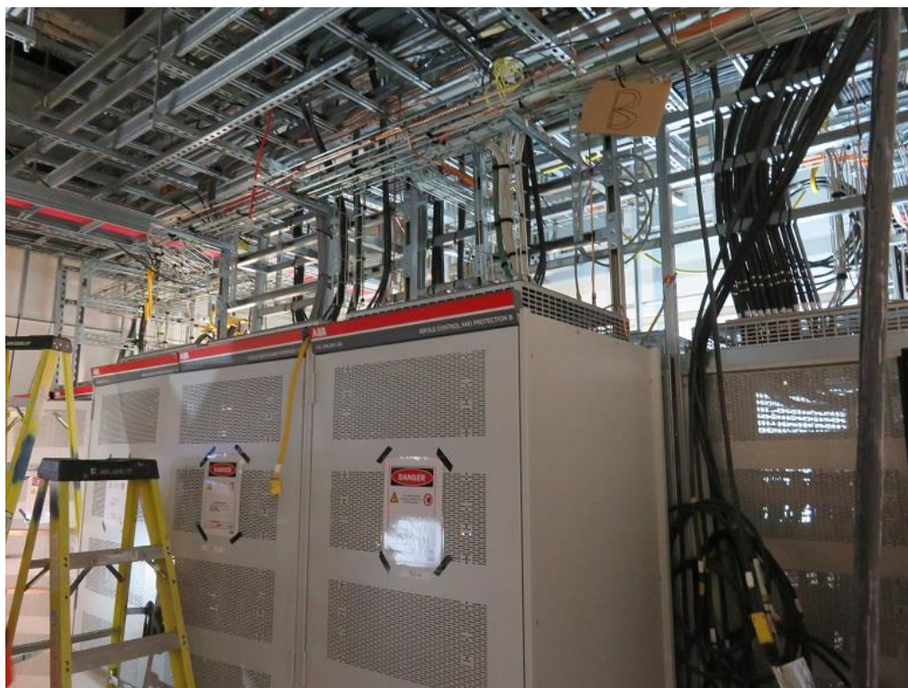
Photo 10: Station control room at Bottom Brook converter building.
