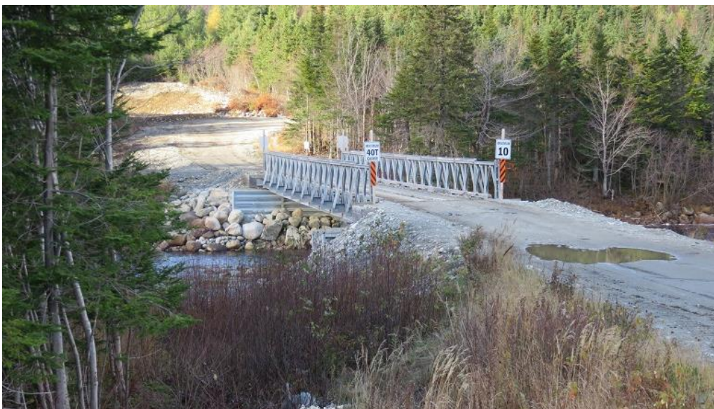
Photo 2: Temporary construction access bridge across Southwest Brook, which is to be removed soon.
