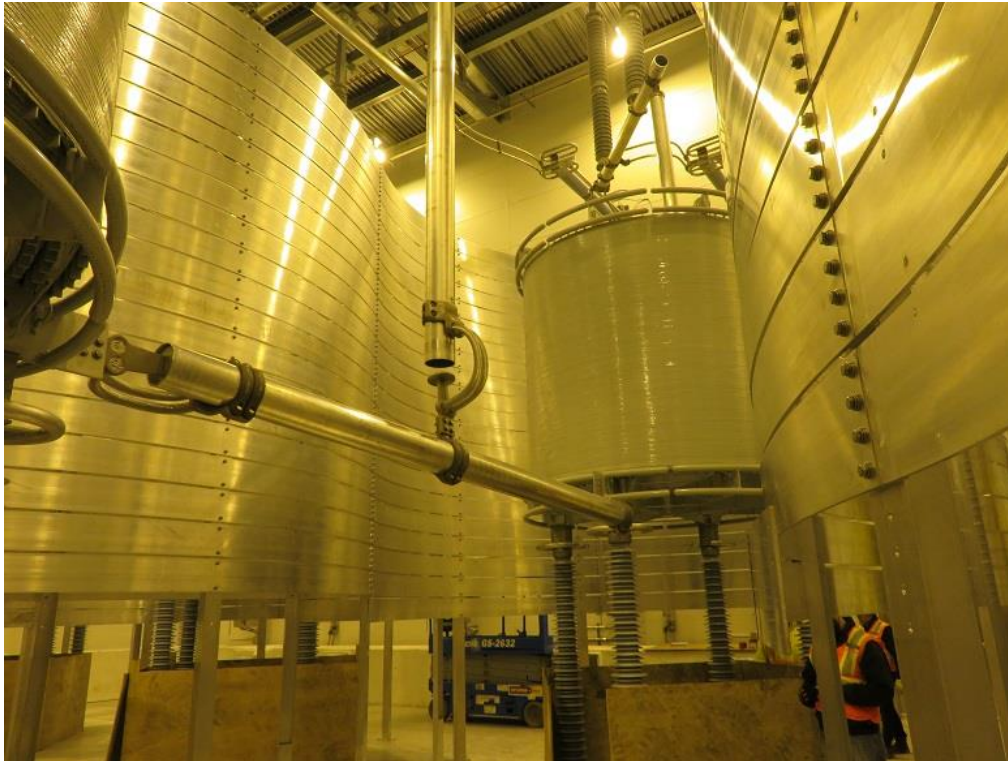
Photo 9: Pole 1 reactor room at Bottom Brook converter building.
