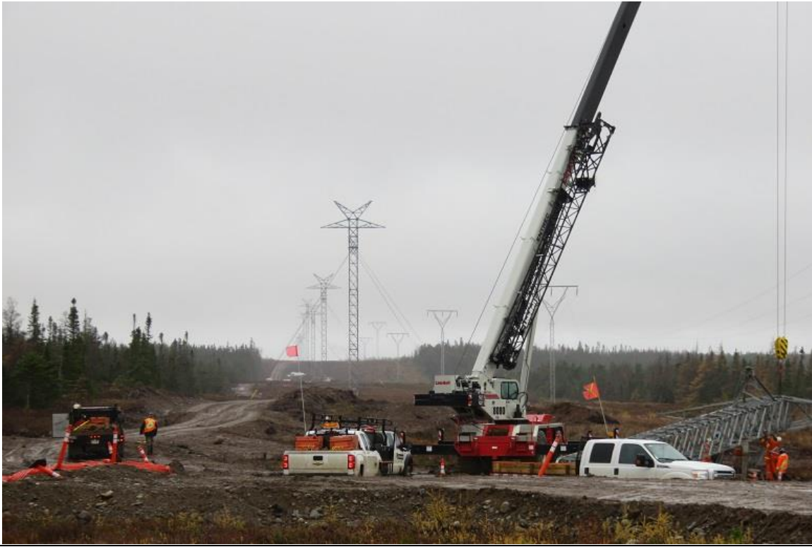
Photo 3: In-progress erection of an HVDC tower. Other completed HVDC towers are in the background at left, and the existing HVAC line is along the right side of the right-of-way.
