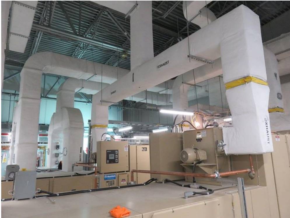
Photo 11: Ventilation equipment at mezzanine floor at Bottom Brook converter building.
