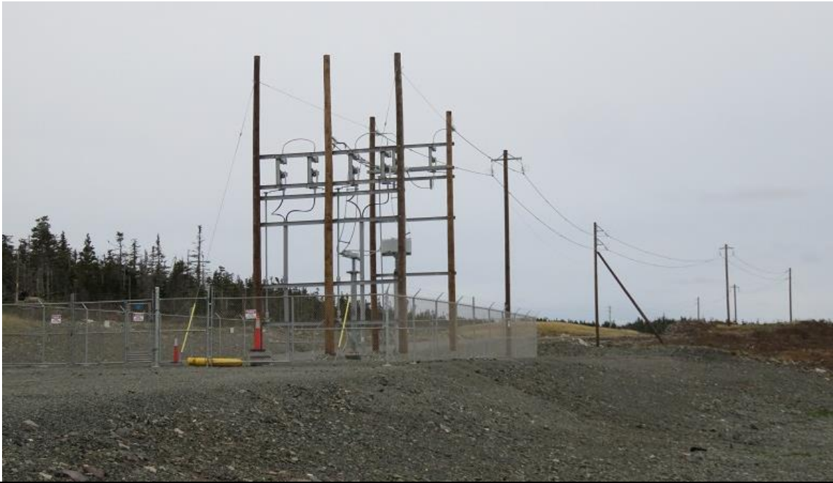
Photo 26: Grounding site at Big Lorraine showing grounding lines transitions from overhead to underground.
