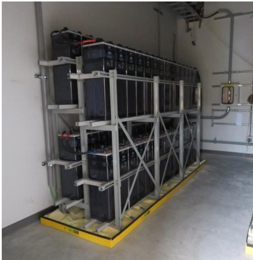
Photo 23: 125VDC battery inside Woodbine converter building are braced and anchored.
