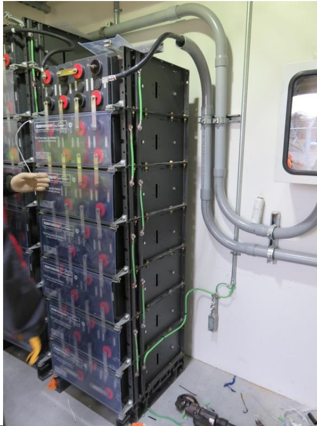
Photo 17: Point Aconi transition compound - Communication battery inside service building is braced and anchored.
