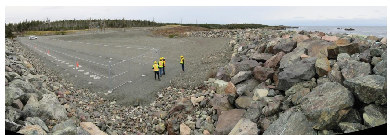
Photo 24: Panorama view inside protective rock berm at Big Lorraine grounding site. Grounding wells with precast concrete covers are located inside the fenced enclosure at left.
