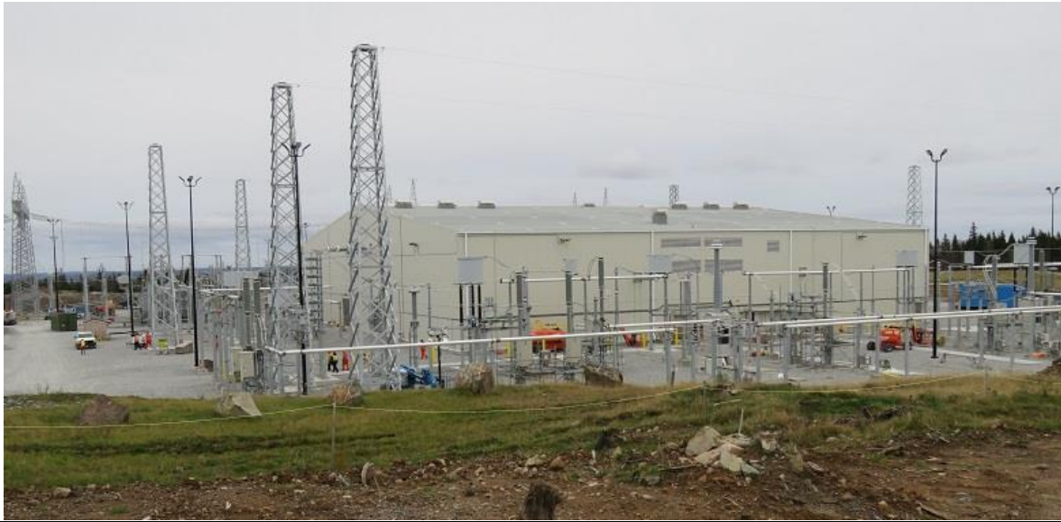
Photo 20: Woodbine converter station.
