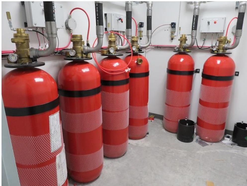
Photo 12: Fire suppression system chemical tanks at Bottom Brook converter building.
