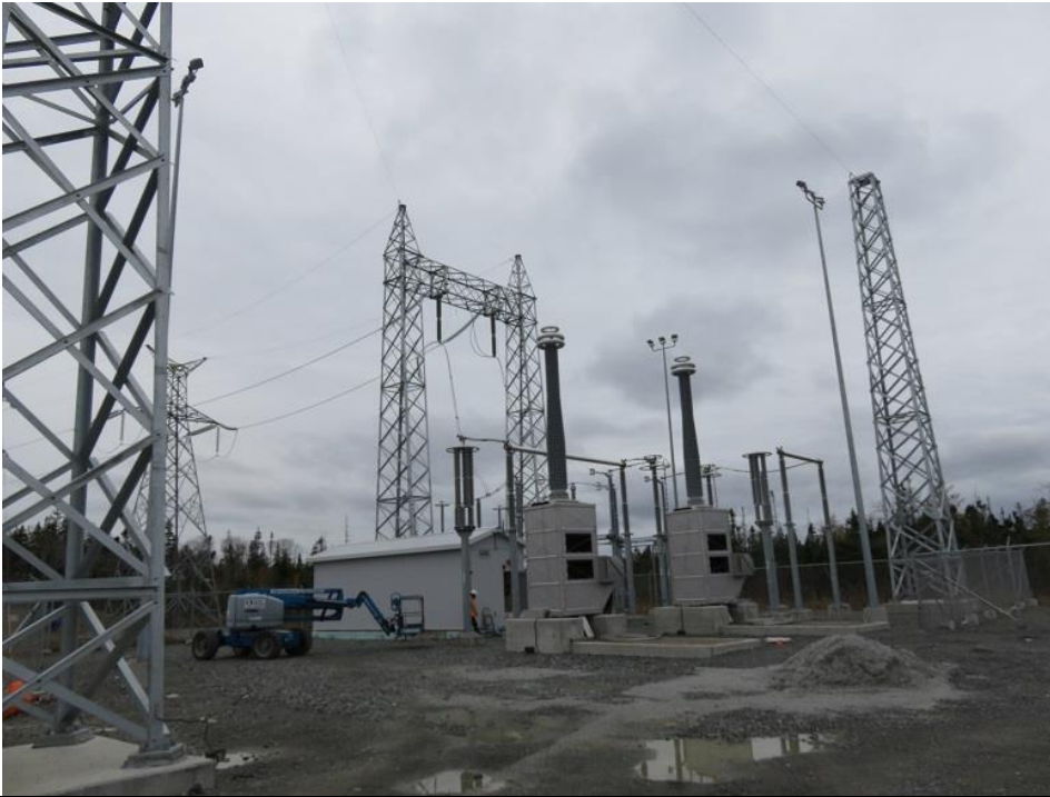
Photo 15: Point Aconi Transition Compound is nearly completed. Overhead connections to the two transition structures in centre of photo are not yet installed. Electrical works are being completed in the service building in background.
