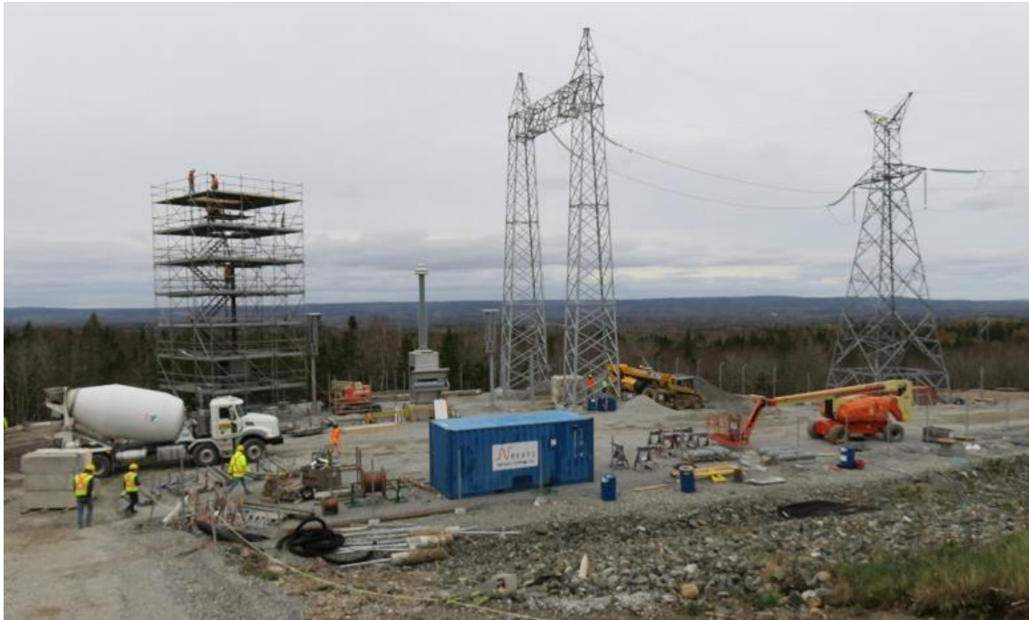
Photo 18: In-progress construction of transition structure where overhead HVDC line transitions to underground on north side of the Woodbine switchyard.
