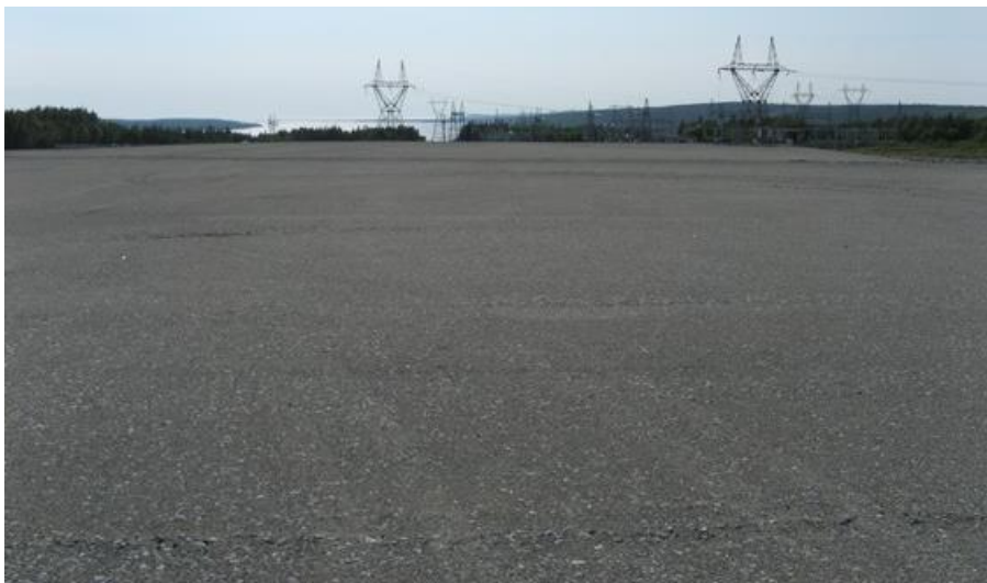
Photo 17 – Bottom Brook - Prepared site for converter station and substation expansion adjacent to existing substation.
