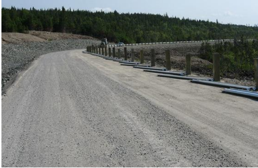
Photo 9 – Indian Head – Finished section of access road, with guard rail installation in progress.
