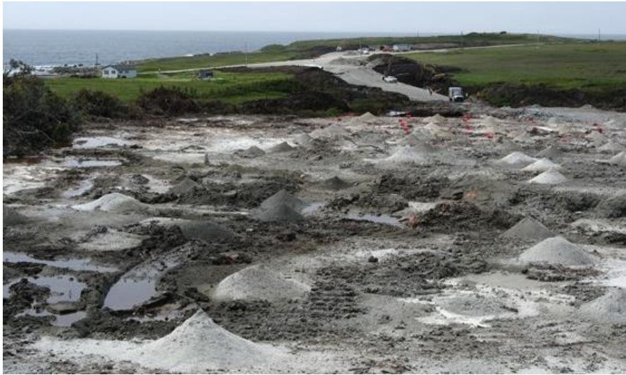
Photo 15 – Cape Ray – Section of bedrock prepared for blasting. The small conical piles are drill cuttings from the holes drilled for explosives.
