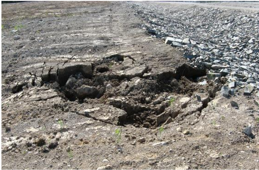
Photo 20 – Bottom Brook – Local depression in waste material adjacent to site, reportedly due to melting of snow that was mixed in.
