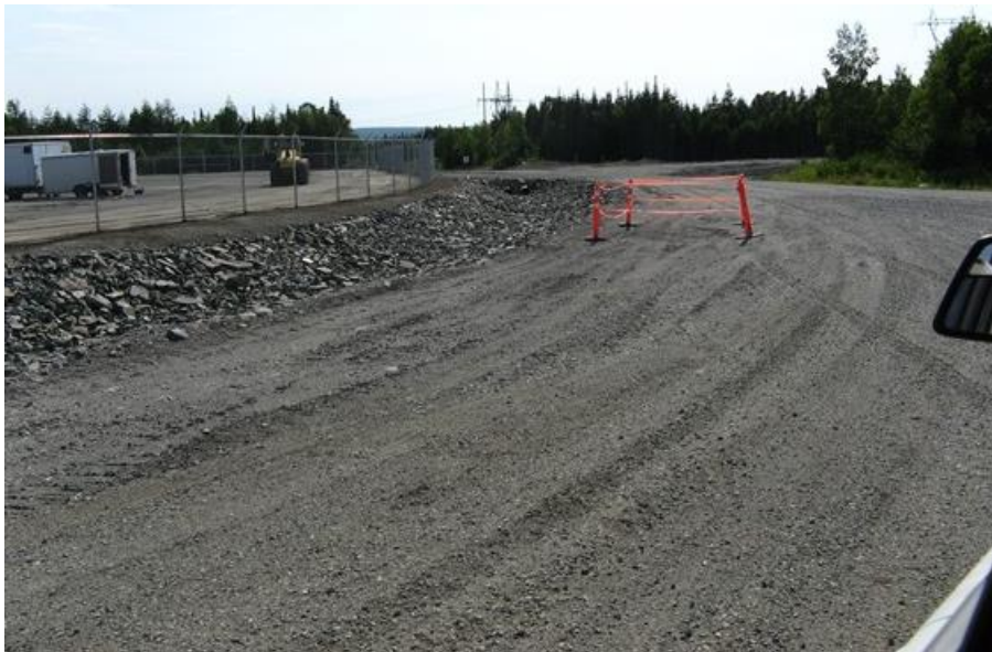
Photo 19 – Bottom Brook – View down access road from location adjacent to existing substation. Fenced marshalling yard is on the left side of photo. Flagged area in the centre of photo is a local sinkhole that requires repair.
