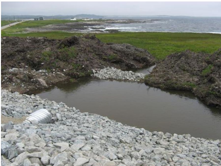
Photo 12 – Cape Ray – Typical settling pond and rock berm for sediment control adjacent to HDD site.
