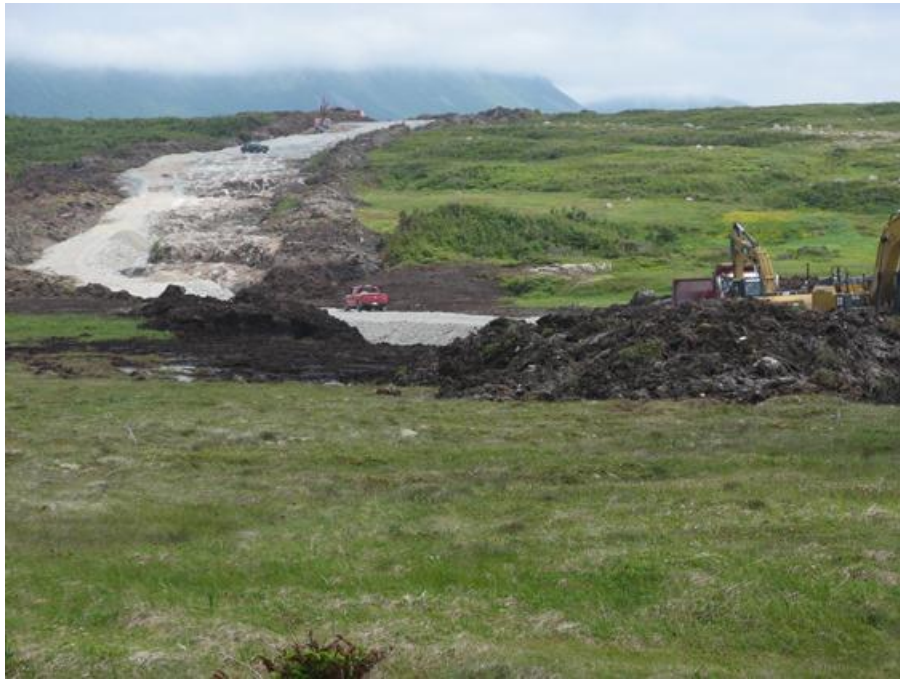
Photo 13 – Cape Ray – View looking up access road being constructed to transition compound.
