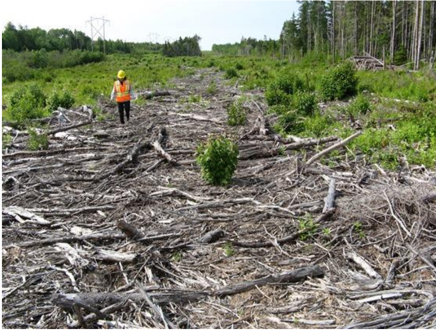
Photo 1 – Point Aconi - View looking southerly along right-of-way from the HDD site to the transition compound.
