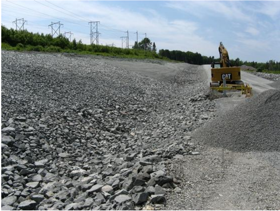
Photo 5 – View up access road to Woodbine transition compound. A security gate is being installed just in front of the excavator.
