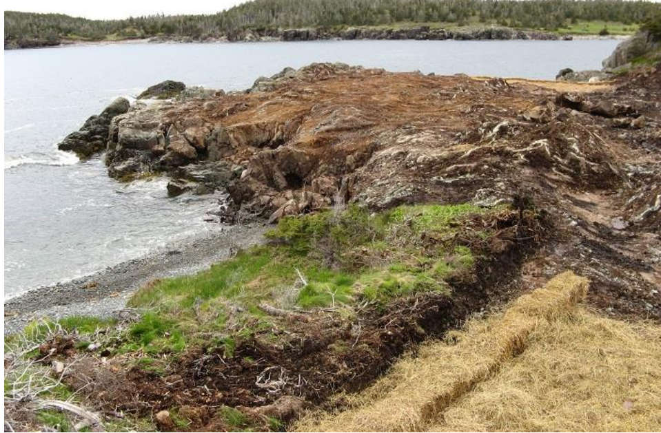
Photo 32 - Access road alignment adjacent to water area where rockfill berm will be constructed.
