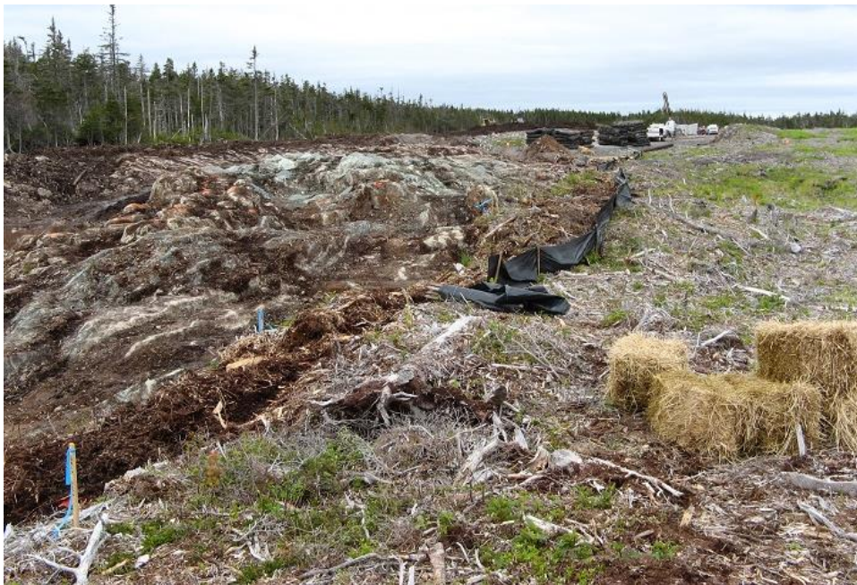
Photo 31 - Access road alignment after stripping of overburden. Silt fences and straw bales are elements of erosion and sediment control. Light grey material in center background is piles of drill cuttings from drilling of blast holes.
