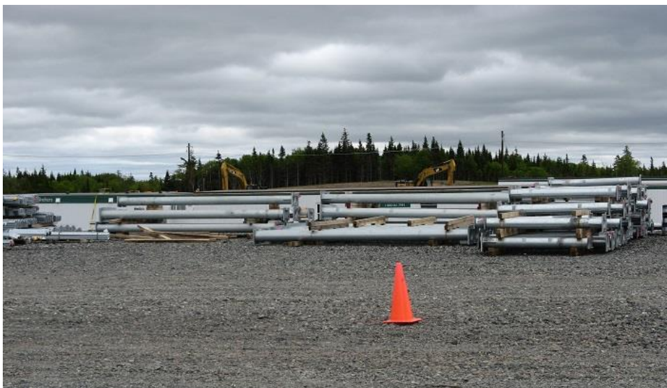
Photo 24 - Components for new DC switchyard.
