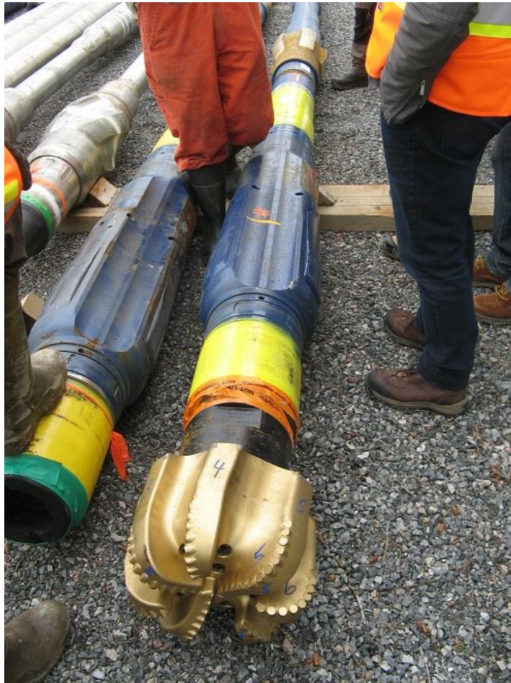
Photo 6 - Drill bit and following drill rod sections. Blue sections contain movable components that are used to steer the drill along its design alignment.
