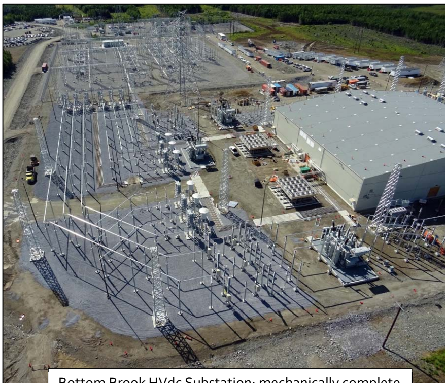
Bottom Brook HVdc Substation: mechanically complete
