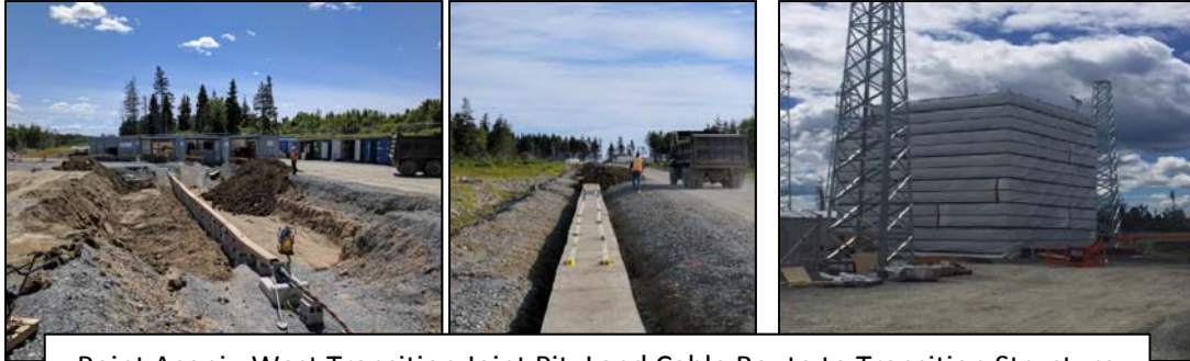
Point Aconi - West Transition Joint Pit, Land Cable Route to Transition Structure
