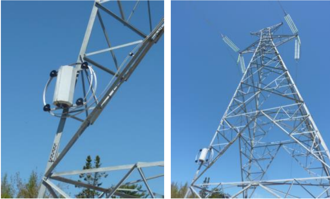
Photos 2 and 3. OPGW Splice Box and transmission tower detail
