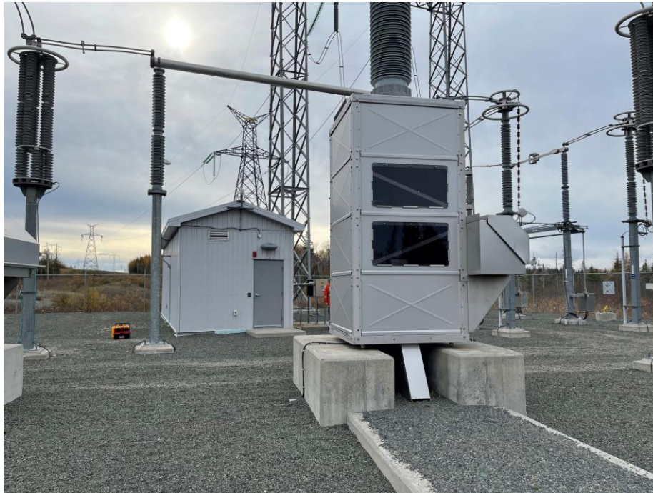
Photo 2: Transition compound – west land cable terminal and control building.
