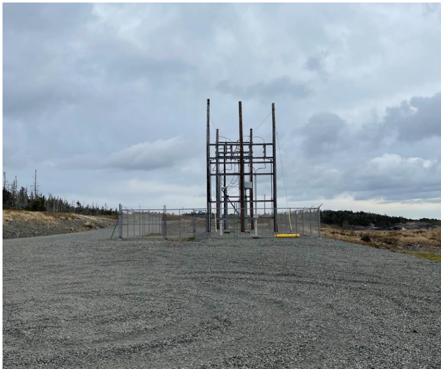
Photo 4: Grounding site - grounding lines transitions from overhead to underground.
