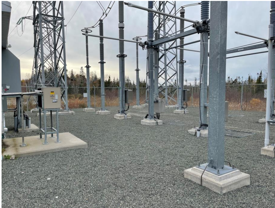
Photo 3: Transition compound – post insulators, disconnect switches and main gantry.
