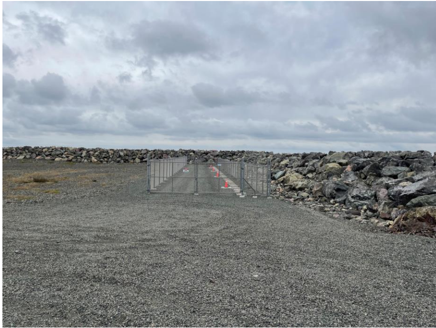
Photo 5: Grounding site - grounding wells with electrodes under precast concrete covers inside the fenced enclosure.
