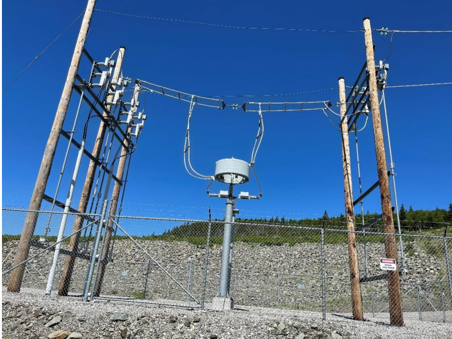
Photo 10: Indian Head grounding line fault detector
