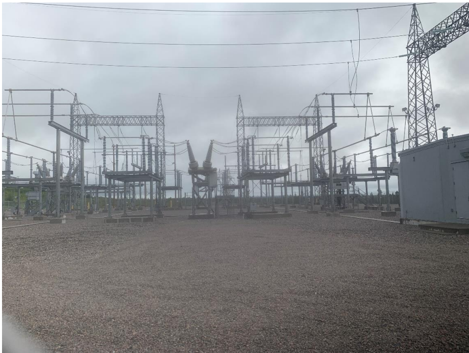
Photo 4: Granite Canal Switching Station
