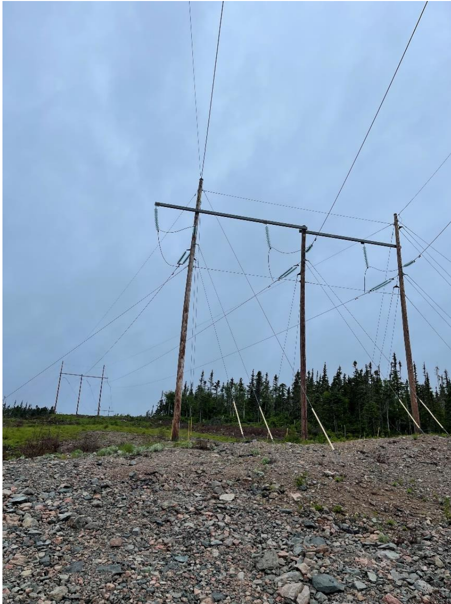
Photo 8: AC transmission line dead-end structure
