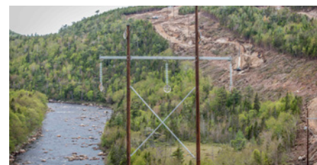
Work continues along the HVac line near the Burgeo Highway in Newfoundland.
