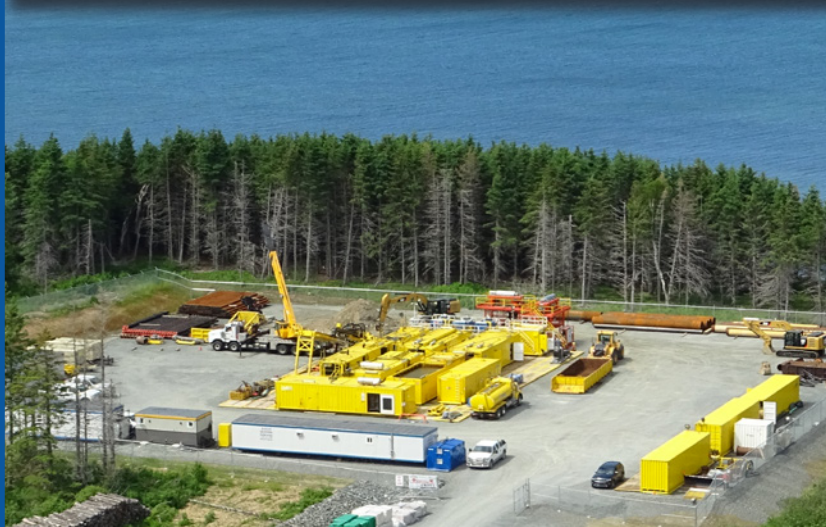
With two HDD boreholes complete at Cape Ray, NL, drilling operations have moved to Point Aconi, NS.
