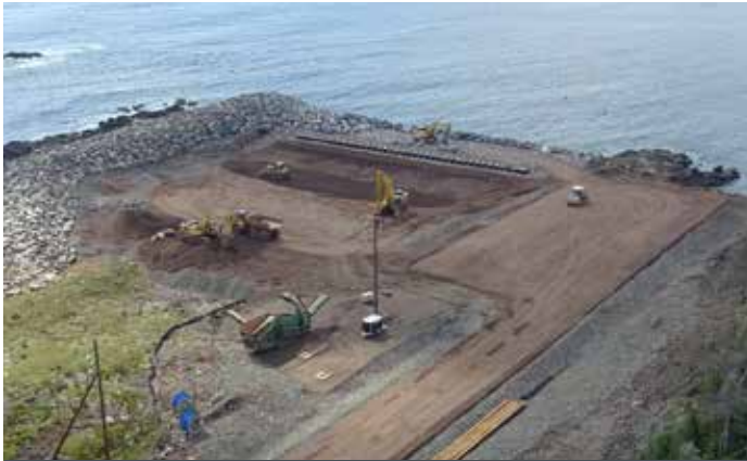
Construction at the grounding site at Big Lorraine, NS, which includes installation of grounding wells.
