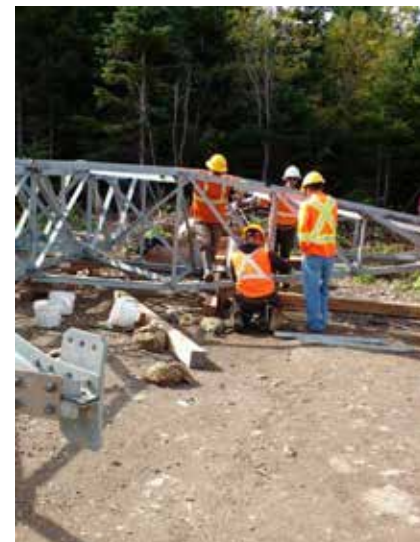
Workers with the Maritime Link Project assembling steel towers along the HVdc route in Nova Scotia.
