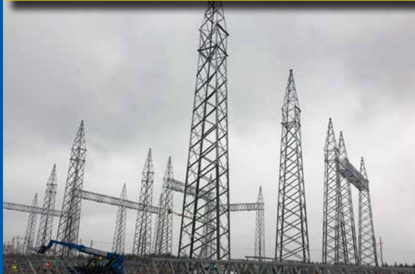
Structural steel work is progressing at the Bottom Brook, NL, and Woodbine, NS, sites.
