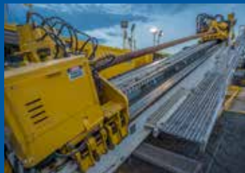
The drill rig used to create boreholes at the Maritime Link Project's landfall sites in NS and NL.
