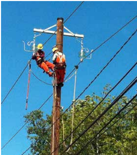
Powerline Technicians work to complete the NS Grounding Line for the Maritime Link Project.
