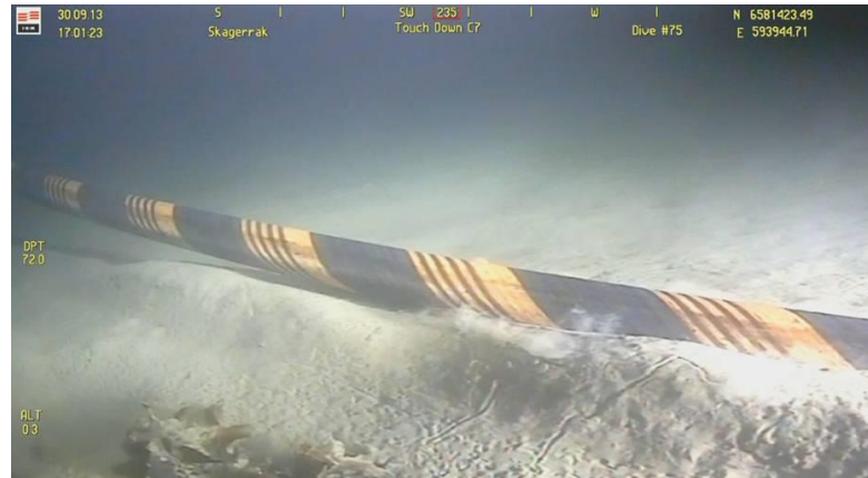
A similar live video will be viewed by the crew onboard the Skagerrak displaying cable laying activity during installation.
